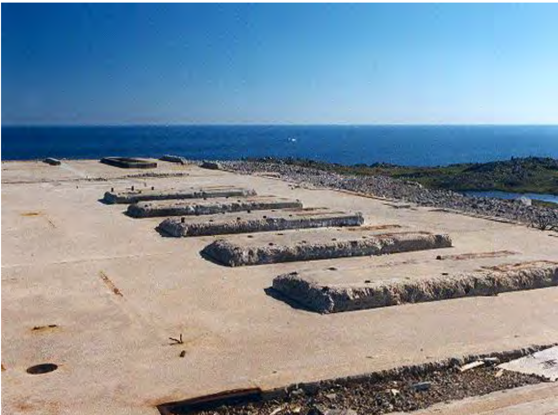
Photo 6: View, looking northeast, following decommissioning activities in area of the former diesel generators - August 2000.
