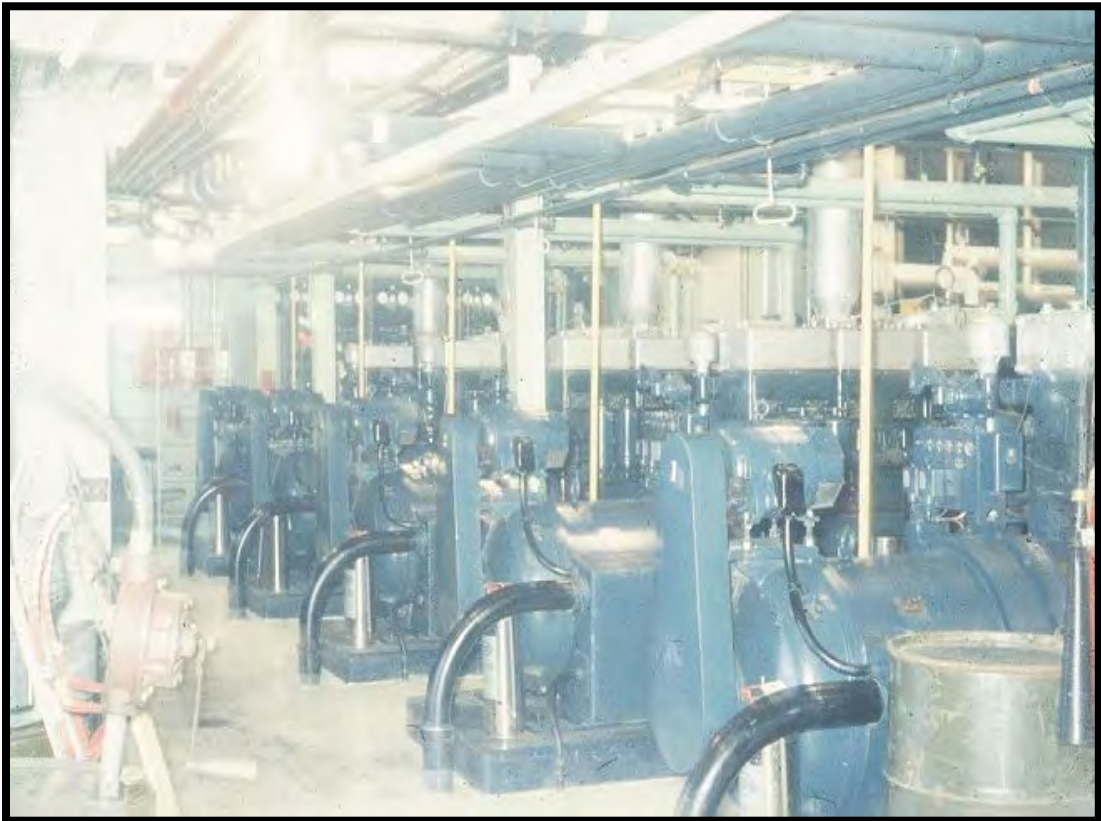
Photo 4: View, looking towards the diesels which supplied the power to the Site - December 1959.
