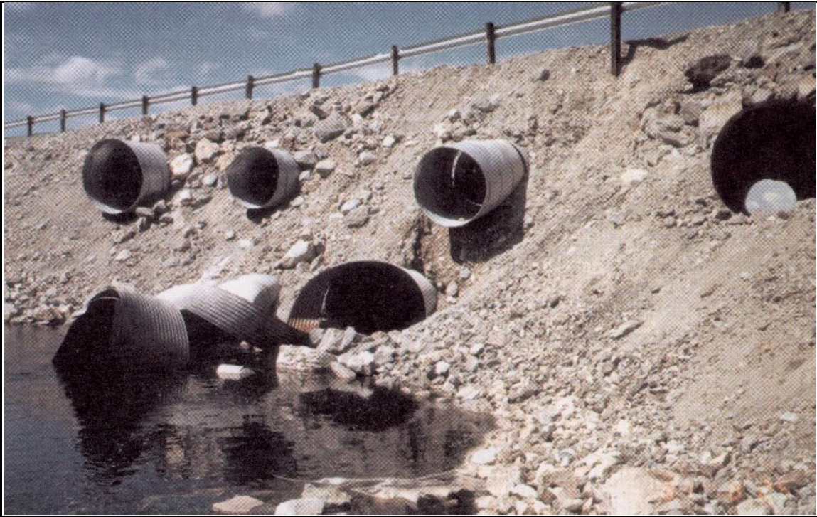
Figure 5.7 Poorly Installed Culverts
