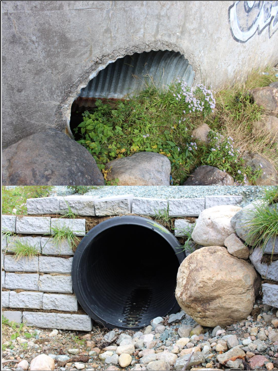
Figure 5.1 A Corrugated Steel Culvert Mitred to the Face of a Wall (Top), and a Small Plastic Culvert with a Masonry Headwall (Bottom)
