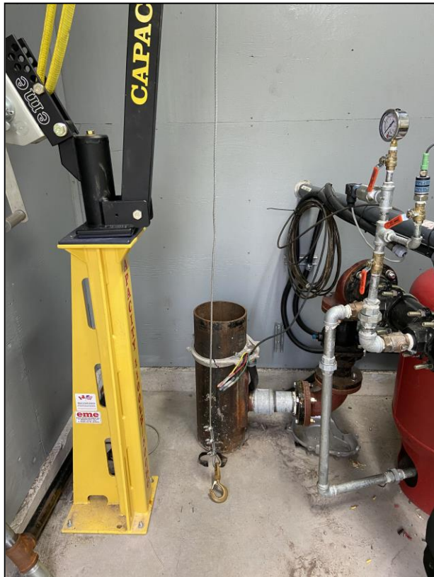
Figure 4: Well Casing in the hut
