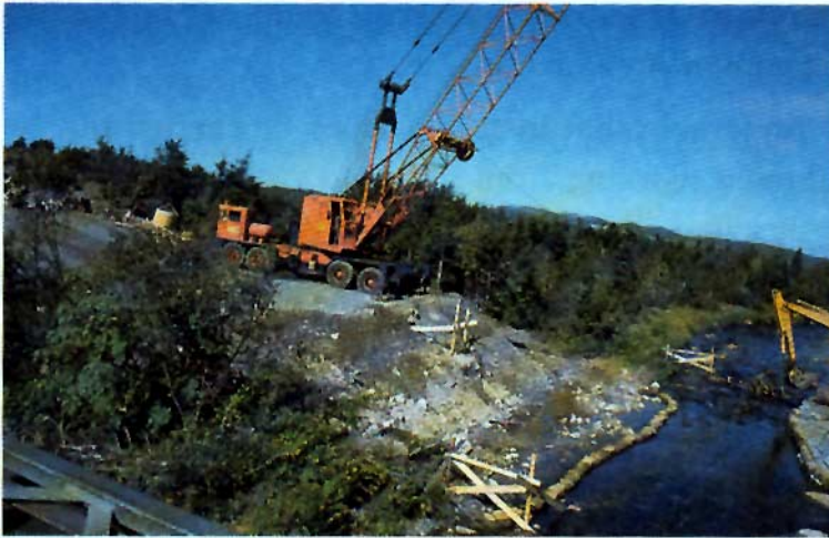
Figure 4.32 Cofferdams can be used to isolate stream margin work areas from stream flow.
