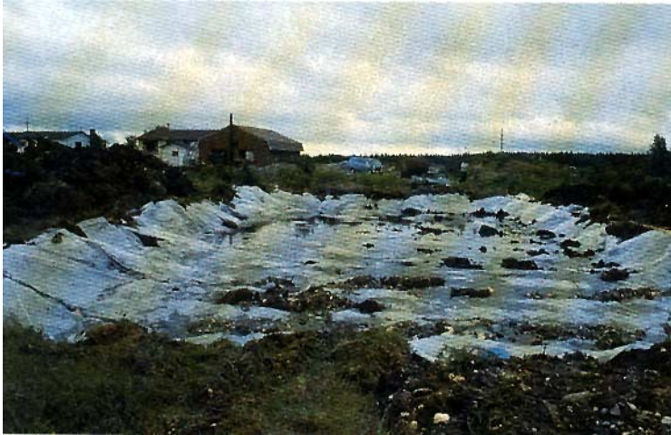
Figure 4.8 Settling ponds should be lined with an impermeable material, such as plastic, to prevent the generation of silt from the excavated settling pond.
