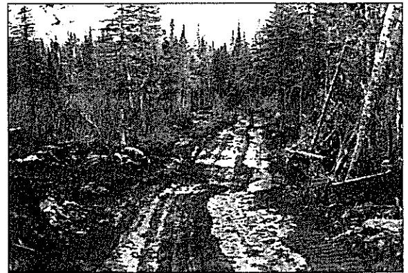
Poorly constructed access road.
