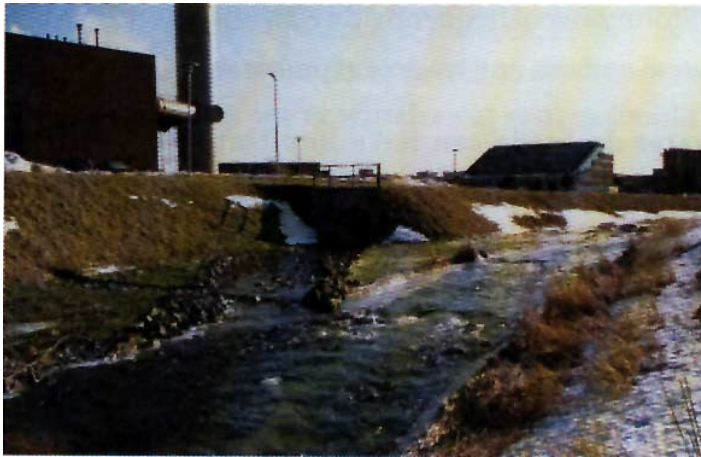
Figure 4.39 Storm drainage outlets should be connected to the receiving watercourse by a channel with orientation parallel to the flow of the receiving watercourse.
