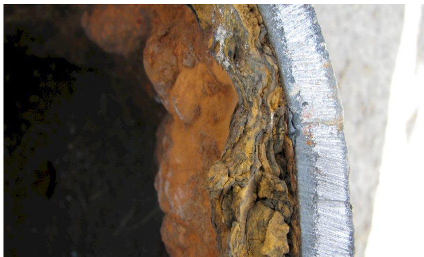
Internal Corrosion (Tuberculation) in Unlined Iron Pipe
