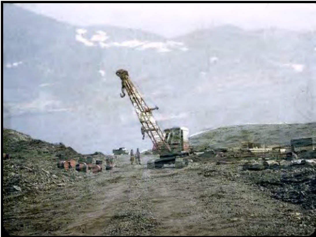
Photo 1: View, looking east, towards the steam shovel used during road construction on the hill near the site circa 1955. Note the POL drums scattered along the roadway.
