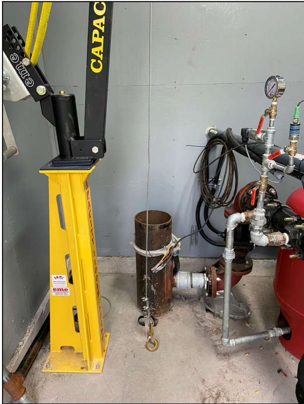
Figure 4: Well Casing in the hut
