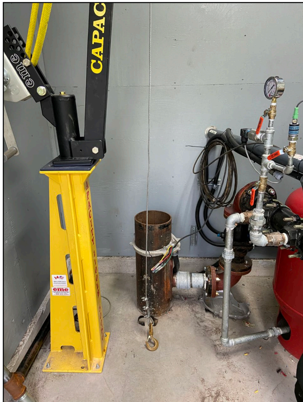
Figure 4: Well Casing in the hut
