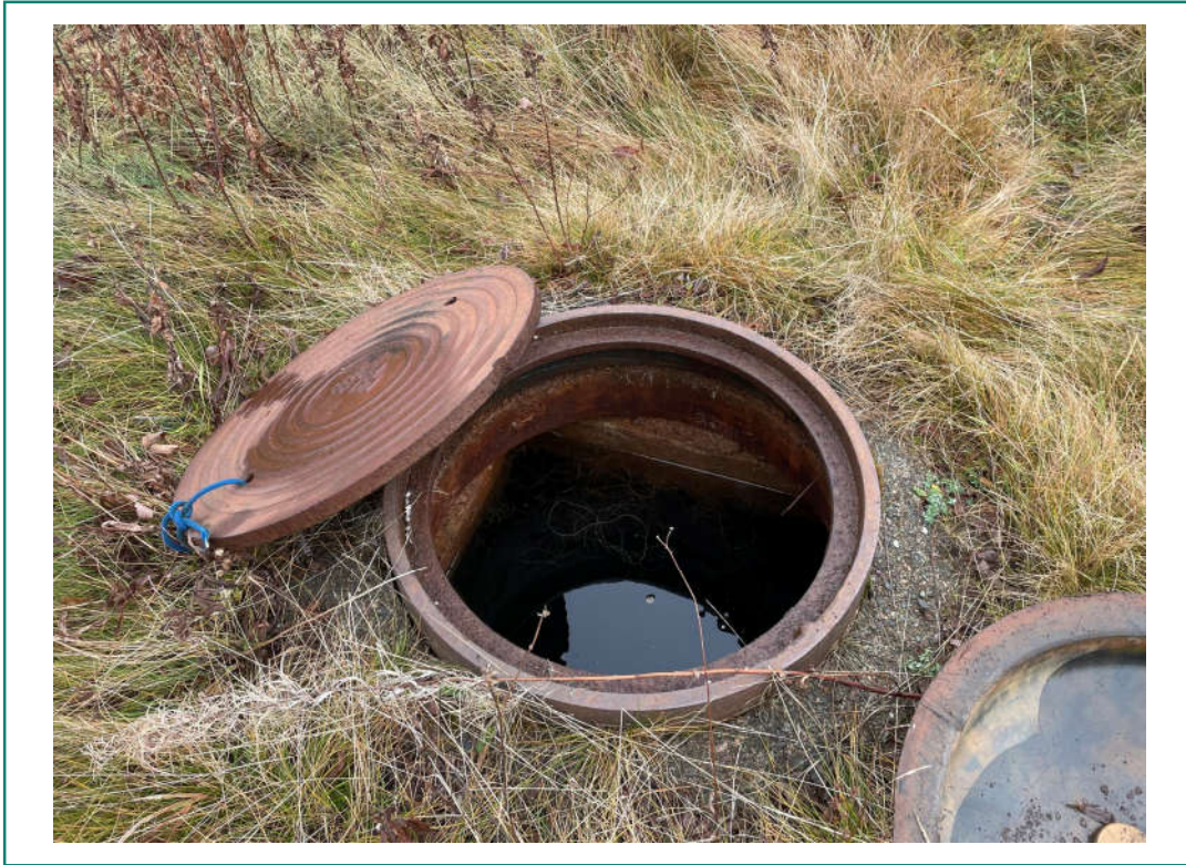
Photo 7: View of the conditions and static water level in the primary liner containment system (PLCS).
