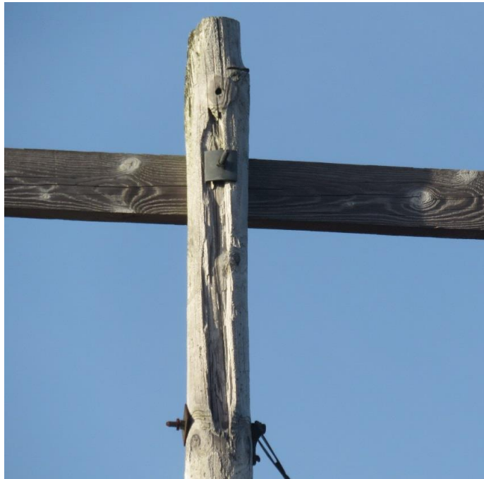
Figure A-1 Deteriorated Pole Top
