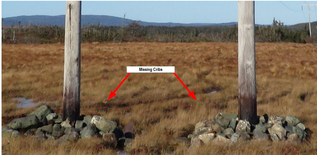
Figure A-9: Missing Cribs
