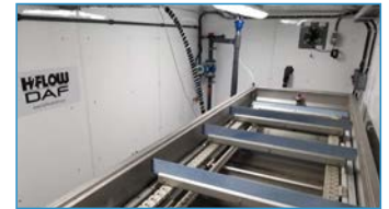
INSIDE A CONTAINERIZED DAF
