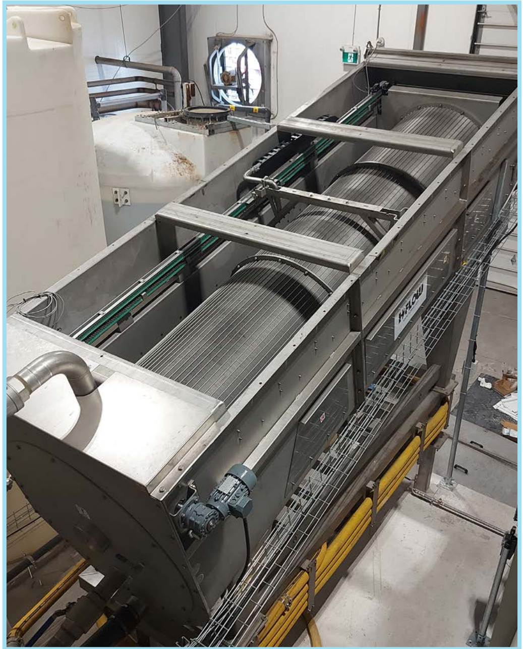
SD SLUDGE SCREW PRESS INSTALLED IN A BEVERAGE COMPANY DAF SLUDGE
