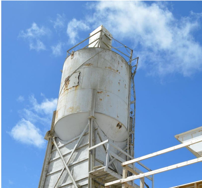
Figure 5. Concrete Batch Plant Silo with Bag House
