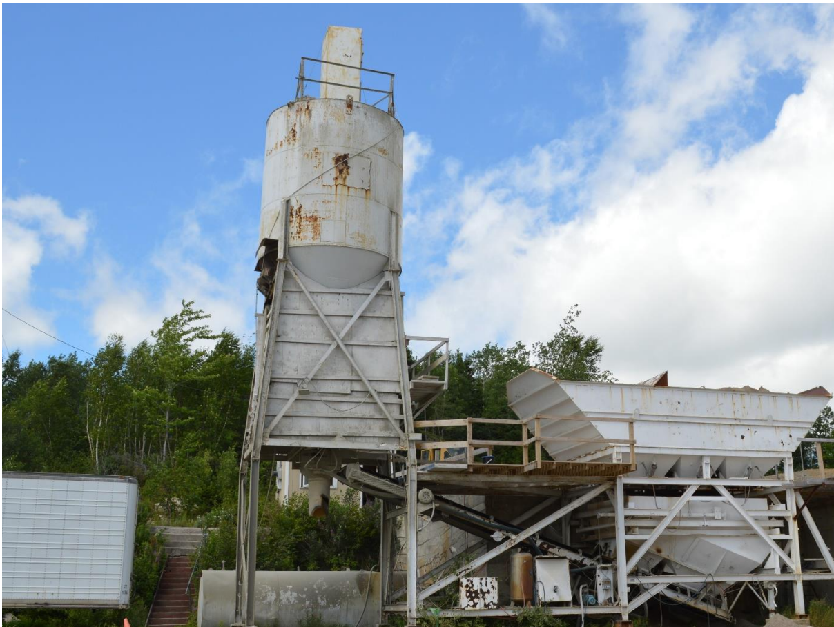
Figure 6. Portable Concrete Batch Plant
