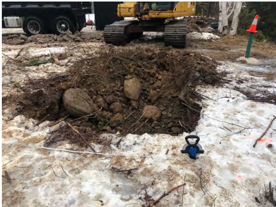
Figure 59. View following the removal of the PAH contaminated soil near the former cableway. Photograph taken February 23, 2022 (GHD, 2022b).
