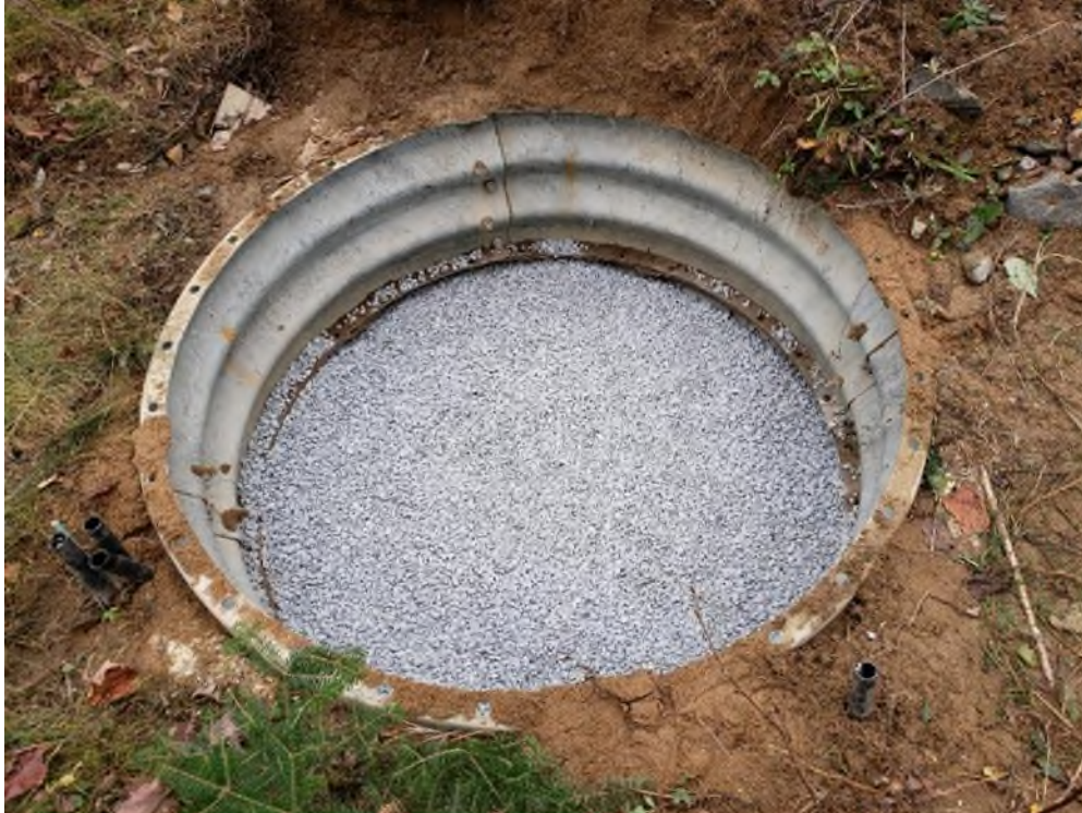
Figure 6. Well filled in with layers of sand and bentonite at 01BP002 (photograph taken October 19, 2021).
