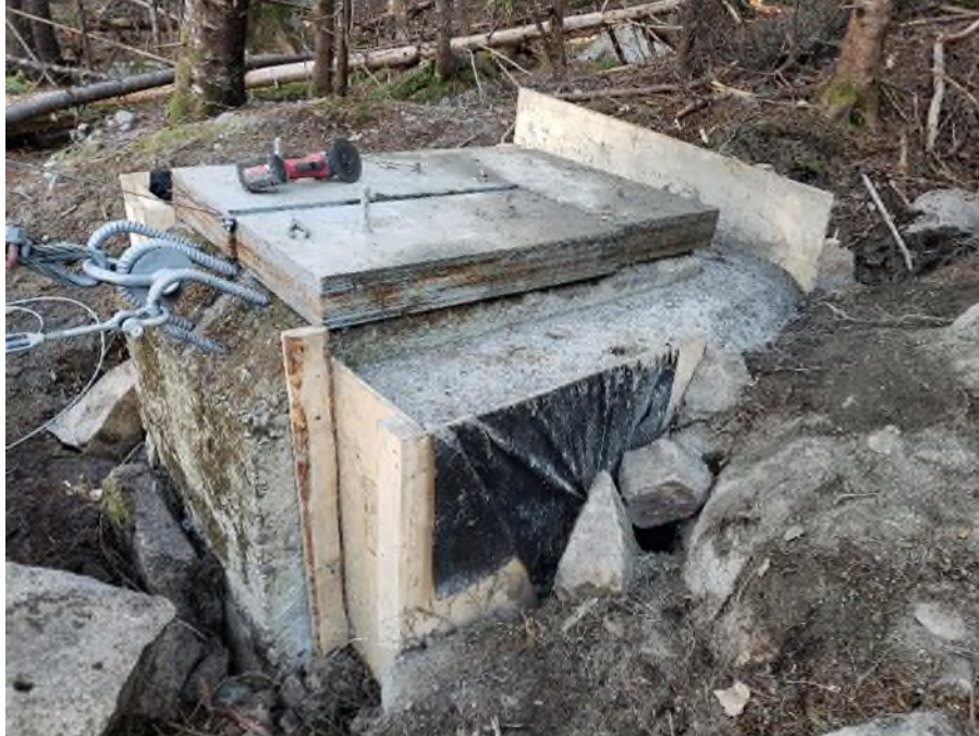
Figure 24. Concrete and steel weight additions to the right bank concrete mass anchor at 01AK001 Shogomoc Stream near Trans Canada (Photograph November 5, 2021).
