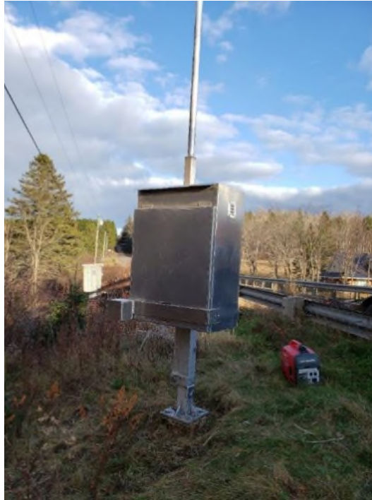
Figure 9. New tilting mast and enclosure at 01BS001 Coal Branch at Beersville (photograph taken November 18, 2020).
