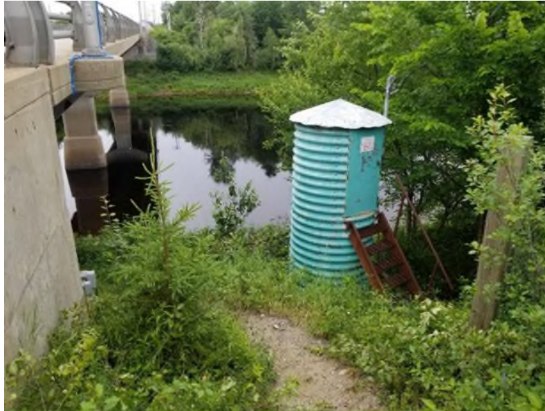
Figure 15. Gauge house and stilling well at 01BO001 Southwest Miramichi River at Blackville (Photograph taken July 23, 2019).
