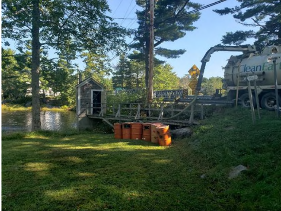
Figure 30. View of sediment being removed from the stilling well prior to decommissioning to be taken to an approved soil handling facility (photograph taken September 22, 2021).
