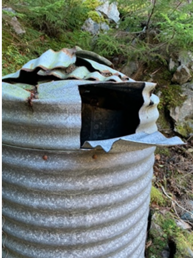
Figure 26. View of stilling well at 01BV006 with access hole cut for sampling purposes (photograph taken November 27, 2021).
