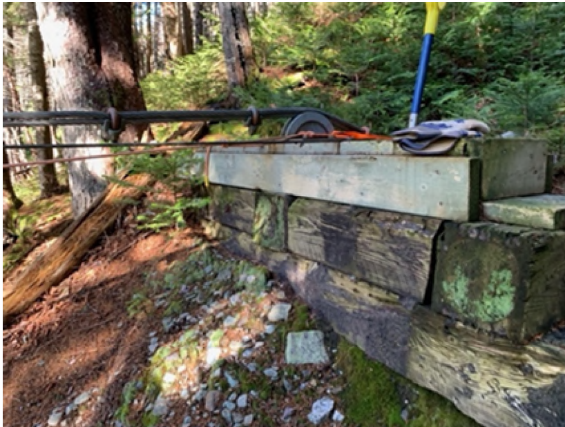
Figure 28. View of creosote-treated cableway timbers on the right bank of the river. Photograph taken mid-November, 2021 (GHD, 2022d).
