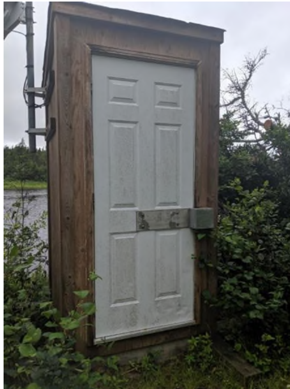
Figure 60. Former walk-in shelter above the stilling well at 02ZK001 Rocky River near Colinet (Photograph taken on July 18, 2019).
