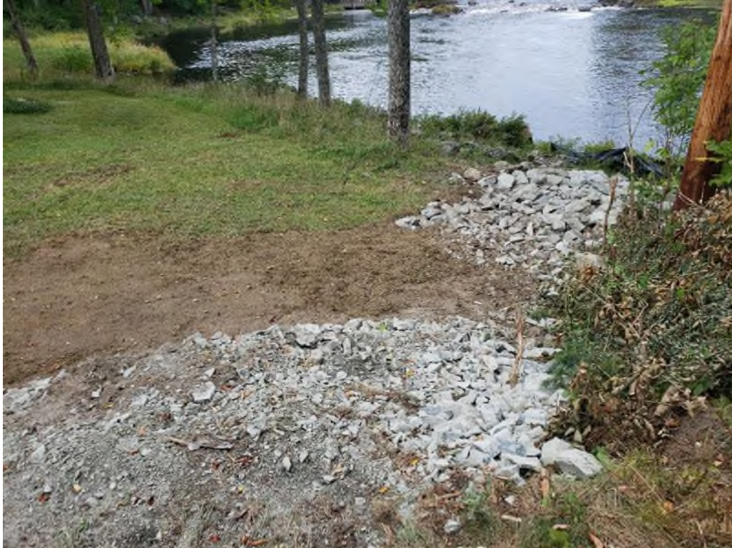
Figure 32. Restored ground where the former 01EE001 hydrometric station was located to match existing land cover (photograph taken September 22, 2021).
