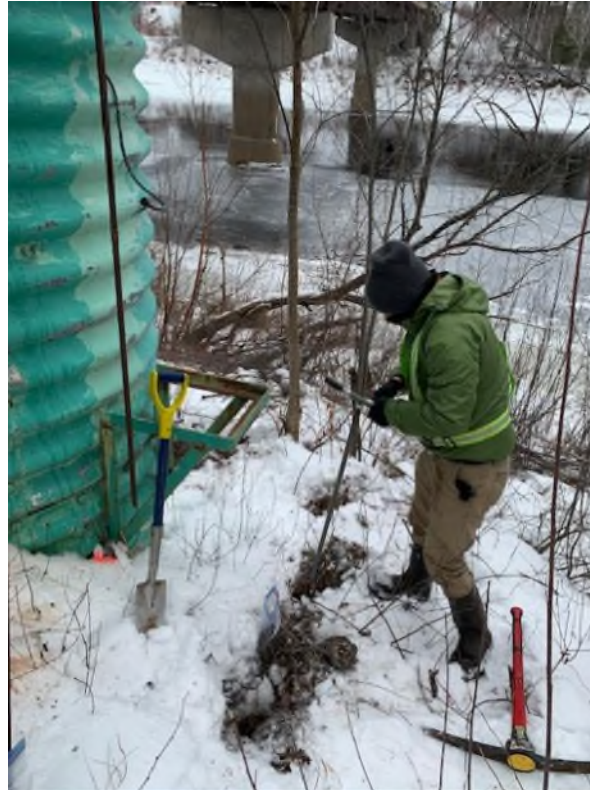
Figure 16. Installation of the shallow monitoring well at 01BO001 by GHD. Photograph taken January 18, 2021 (GHD, 2021b).
