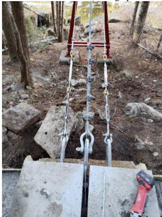
Figure 25. New hardware on the cableway backstays on the right bank at 01AK001 Shogomoc Stream near Trans Canada (Photograph November 5, 2021).
