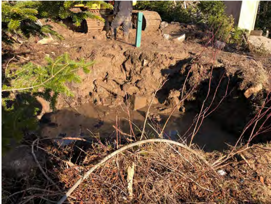
Figure 62. View following the removal of the potentially contaminated soil around the former stilling well. Photograph taken February 10, 2022 (GHD, 2022f).
