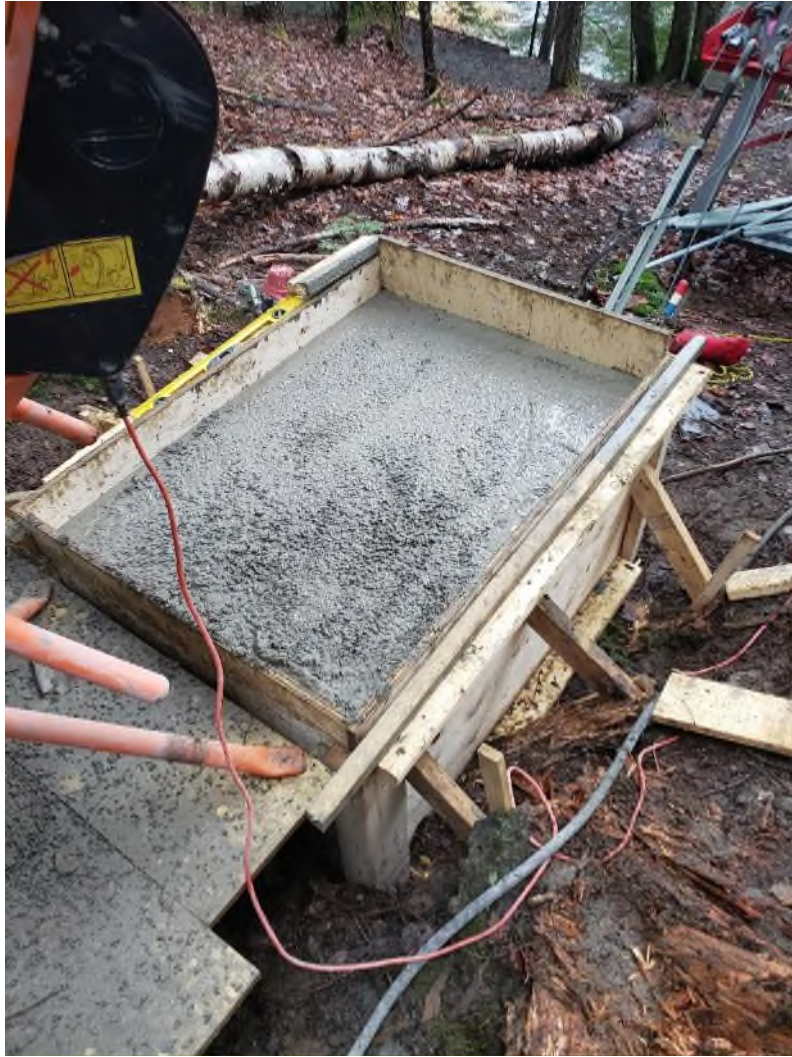
Figure 36. Additional mass added to the cableway anchor system on the left bank (photograph taken November 19, 2021).
