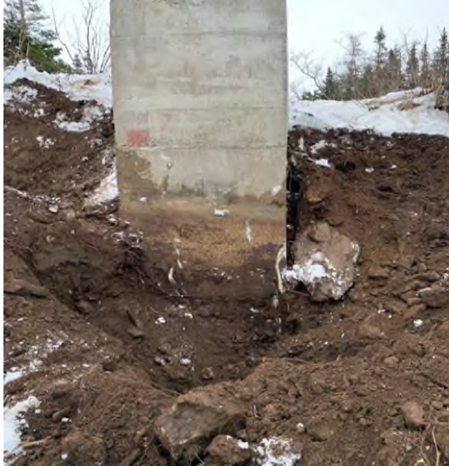
Figure 53. View looking south of the excavation of the concrete stilling well. Photograph taken February 9, 2022 (GHD, 2022e).
