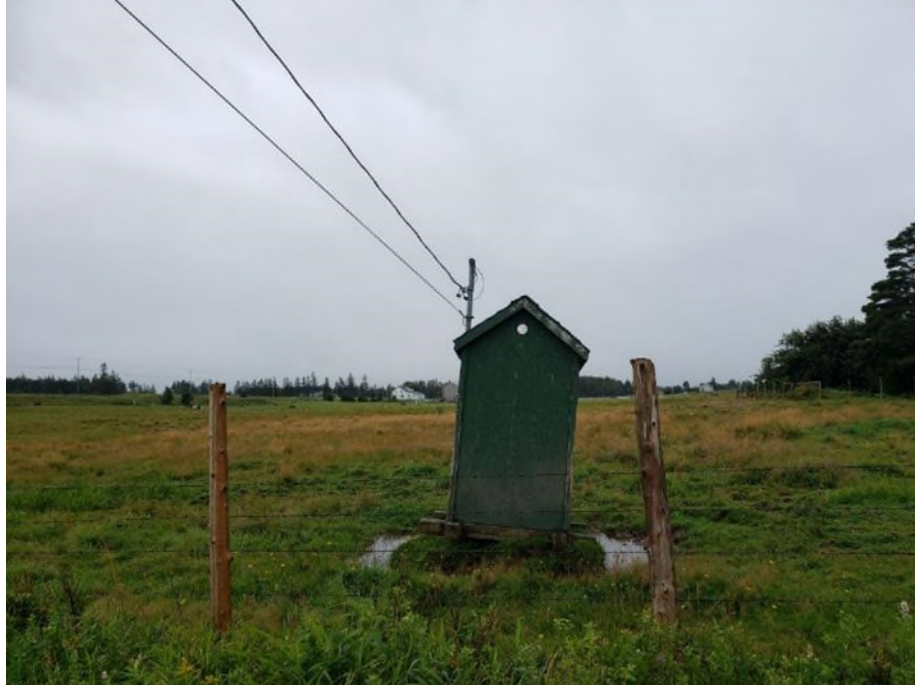
Figure 20. View of tilting shelter at 01BTG02 prior to improvements (photograph taken August 6, 2021).
