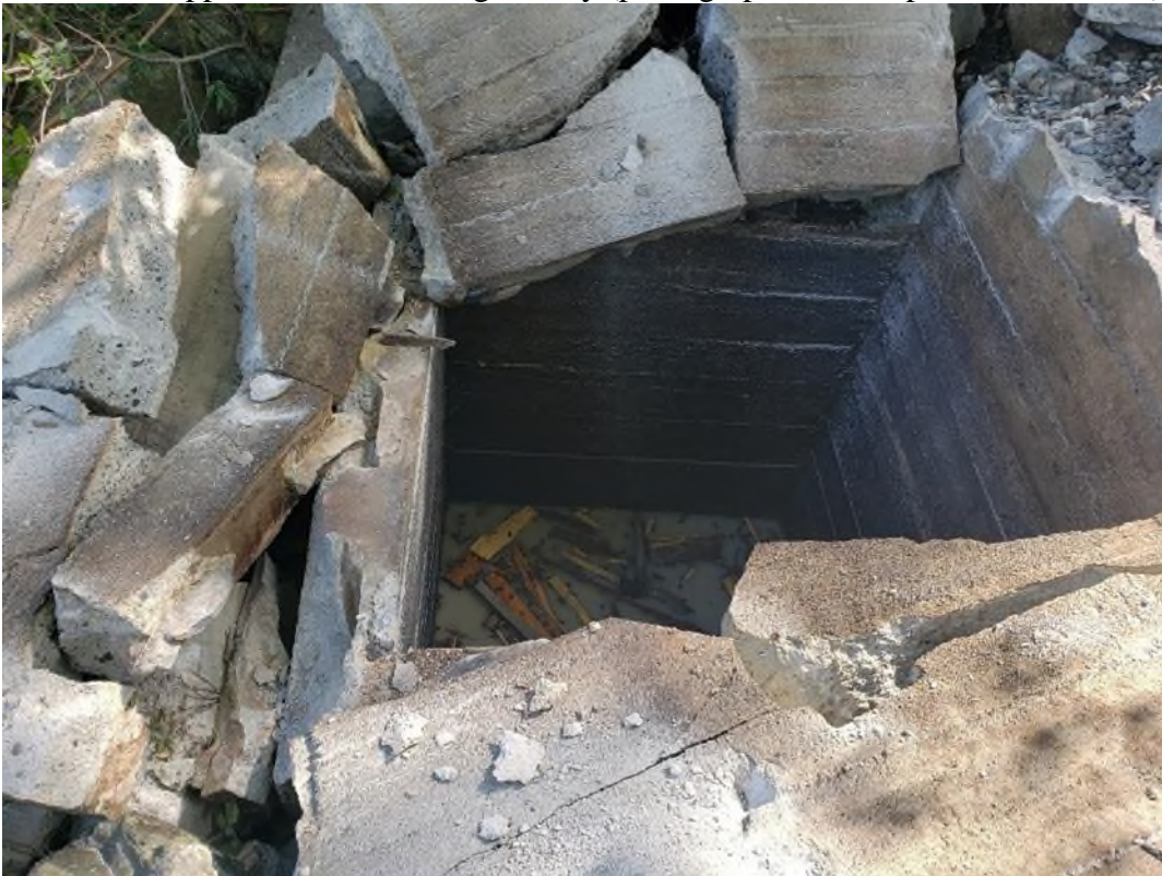
Figure 31. View of the broken well casing during the decommissioning (photograph taken September 22, 2021).
