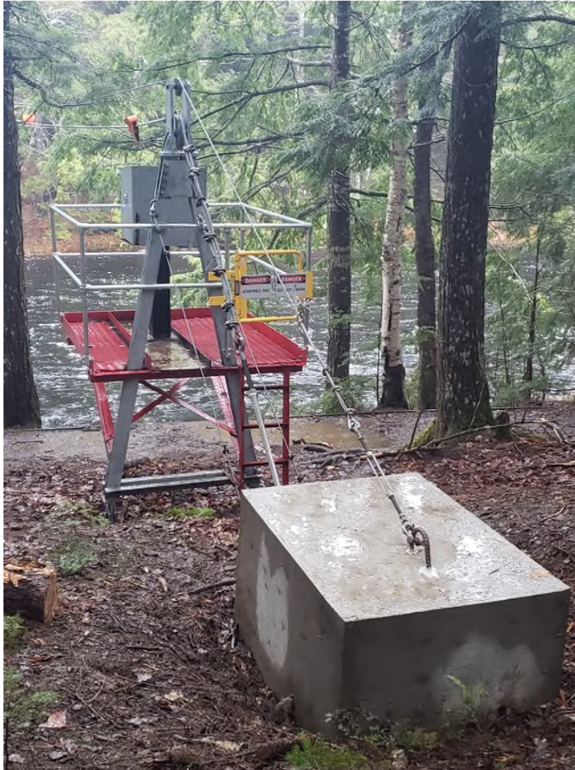
Figure 39. View of the renovated BOC at 01ED007 Mersey River below Mill Falls on the left bank (Photograph taken November 19, 2021).
