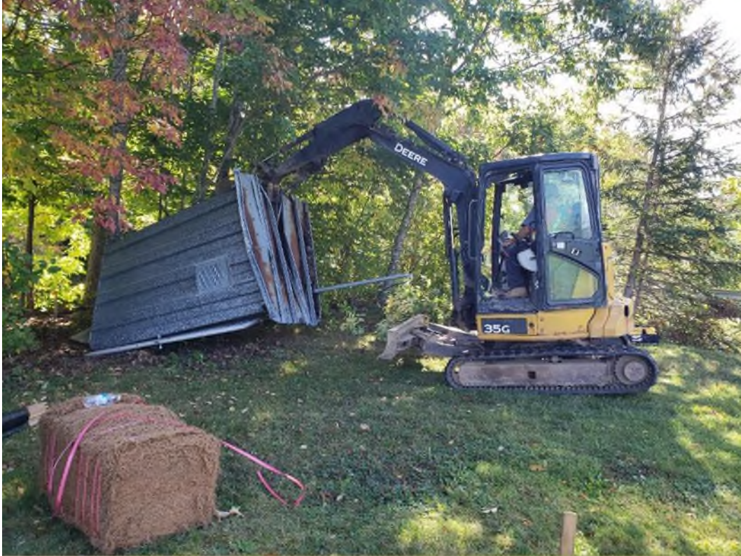
Figure 42. View of the removal of the shelter during the decommissioning at 01DP004 (photograph taken September 27, 2021).
