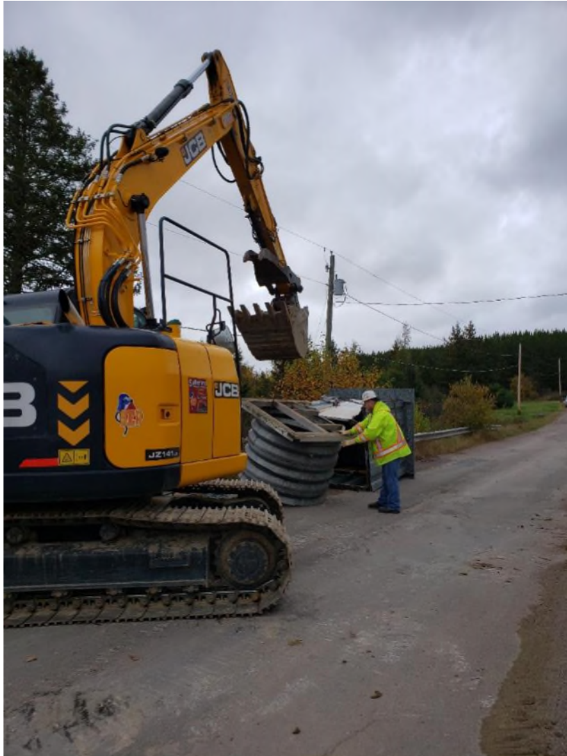
Figure 13. Shelter and well casing being removed from the site (photograph taken October 20, 2021).
