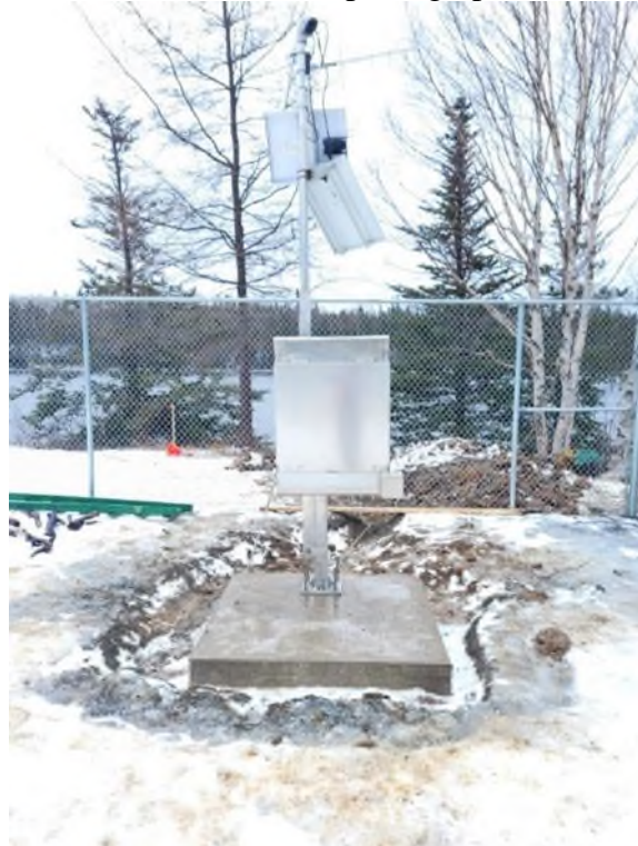
Figure 56. Look-in shelter and pre-cast concrete pad at 01YO011 (photograph taken February 23, 2022).
