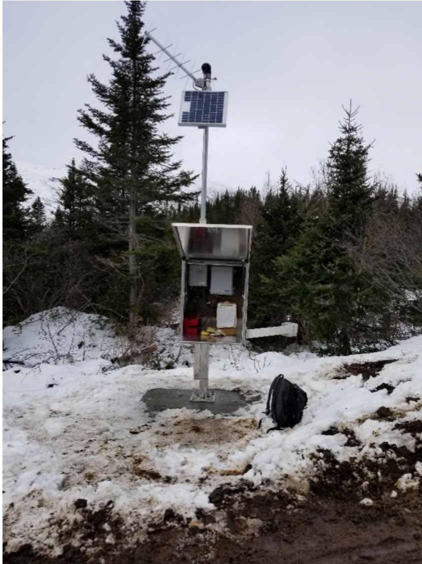
Figure 52. New aluminum tilting mast style look-in shelter installed on a pre-cast concrete pad at 02ZB001 Isle aux Morts River below Highway Bridge (Photograph taken February 10, 2022).
