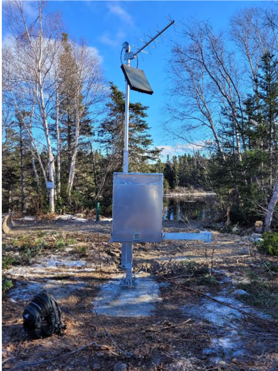
Figure 66. New aluminum tilting mast for look-in style shelter at 02YS005 Terra Nova River at Glovertown installed on the former cableway concrete mass anchor (Photograph taken February 1, 2022).
