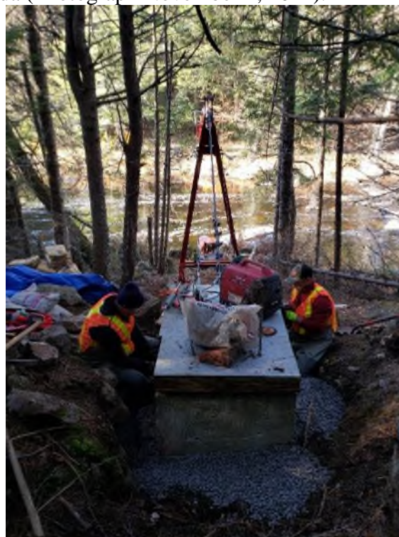
Figure 23. Constructing concrete formwork to upgrade the right bank mass anchor at 01AK001 Shogomoc Stream near Trans Canada (Photograph November 3, 2021).
