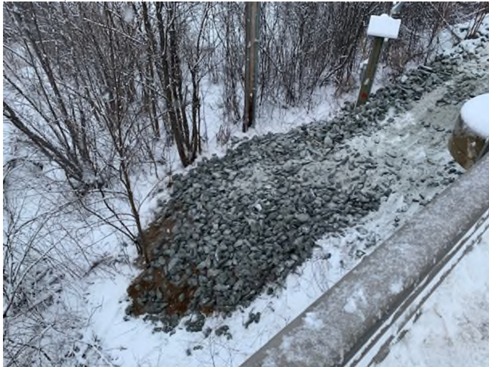
Figure 19. View of well and remedial area grading with rock. Photograph taken January 12, 2022 (GHD, 2022a).
