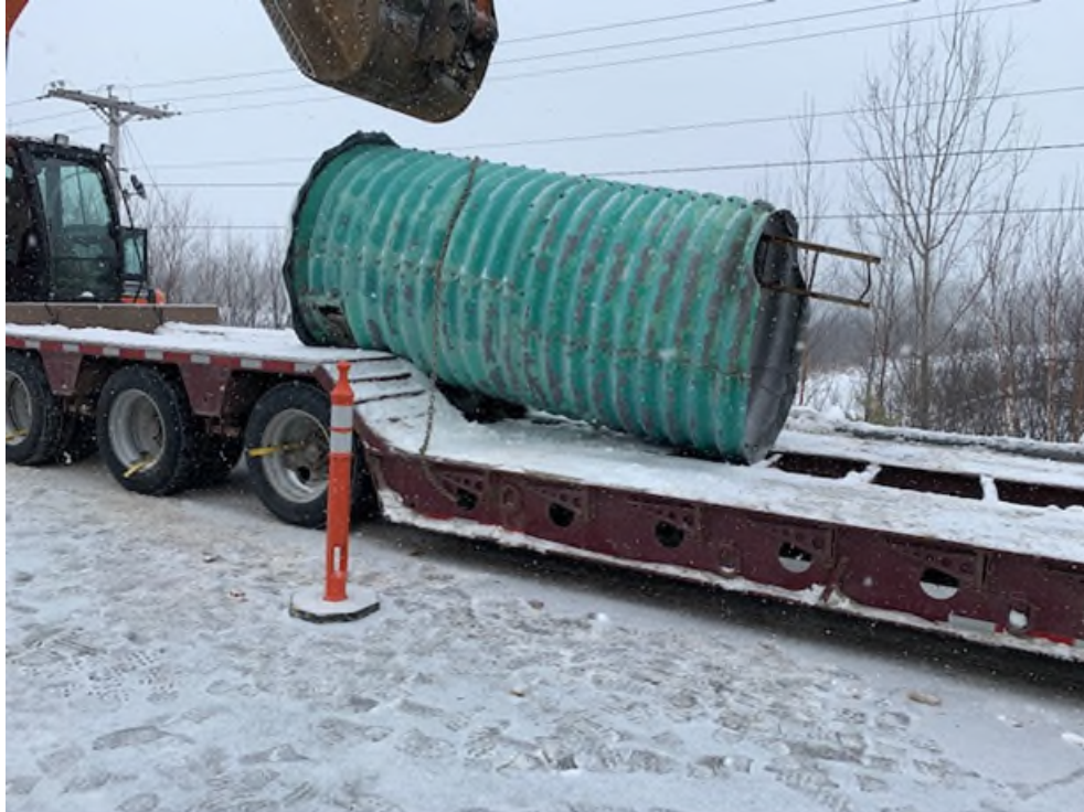
Figure 18. View of the removal of the station well top at 01BO001. Photograph taken January 12, 2022 (GHD, 2022).
