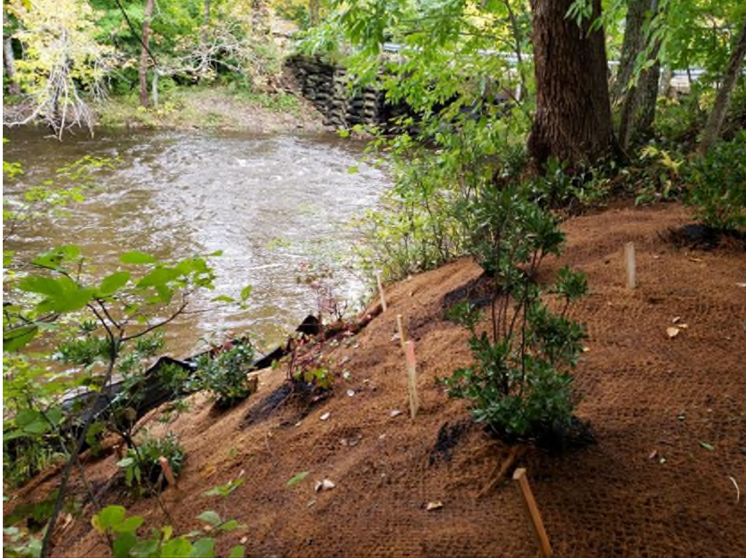
Figure 43. Restored and stabilized bank with native vegetation (Bayberry, Summer Sweet and Red Osier Dogwood) at 01DP004 after well was cut below grade and filled in (photograph taken September 29, 2021).
