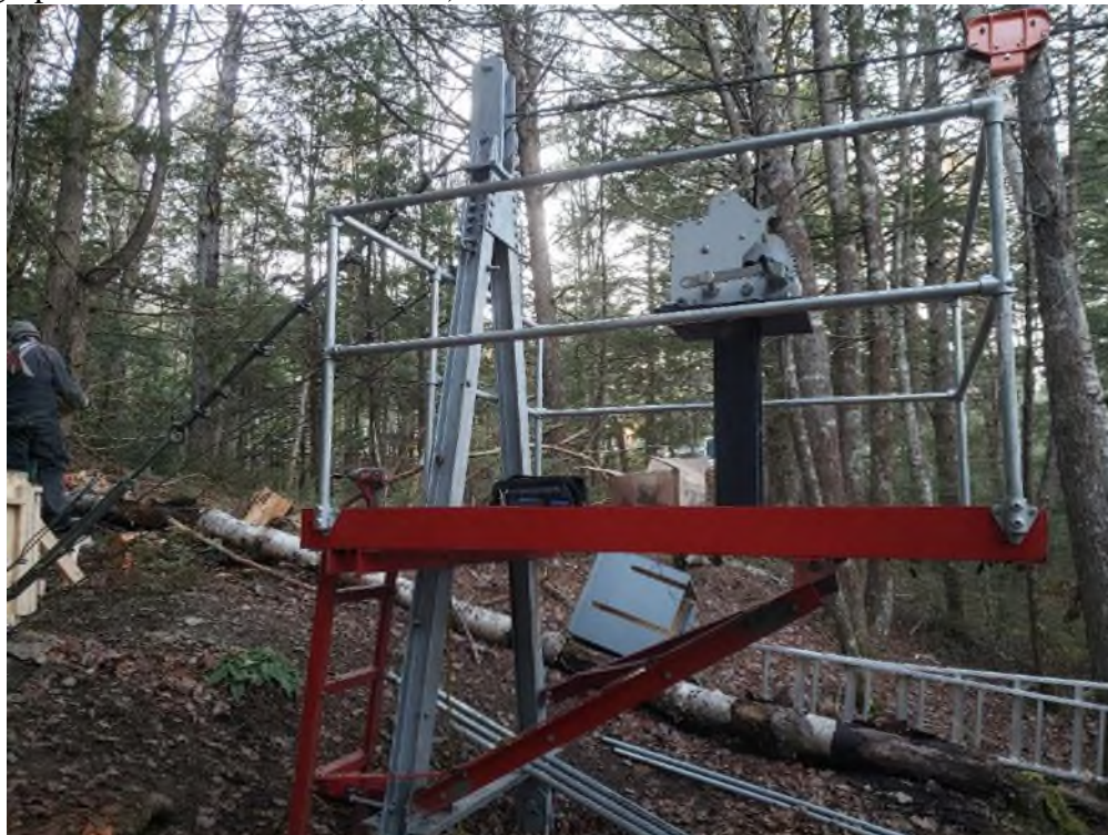
Figure 38. View of the railing added to the cableway platform on the left bank (photograph taken November 19, 2021).
