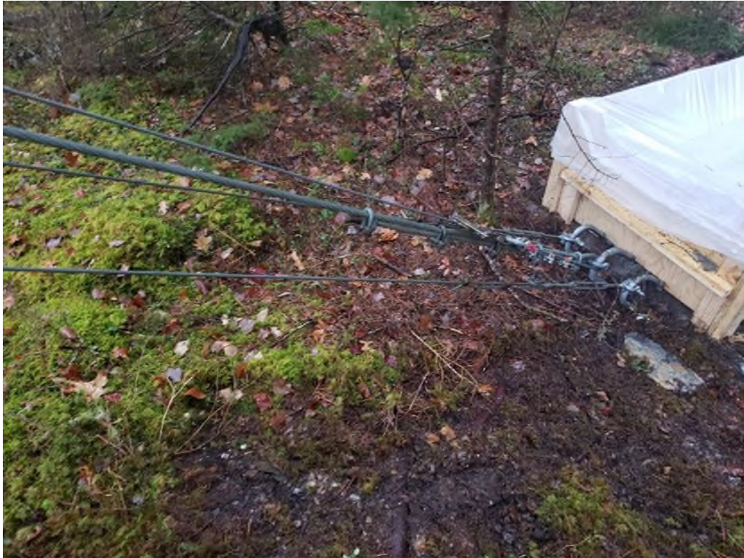
Figure 37. Additional mass added to the cableway anchor system on the right bank (photograph taken November 19, 2021).
