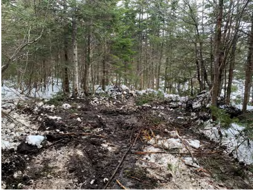
Figure 54. View of the north side of the river following the backfilling of the area of the former A-frame of the cableway. Photograph taken February 10, 2022 (GHD, 2022e).
