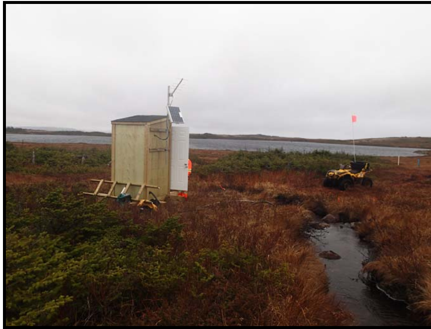
Figure 2: Real-Time Water Quality and Quantity Station at Outflow of Grebes Nest Pond.
