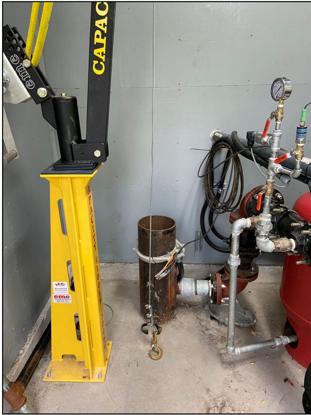
Figure 4: Well Casing in the hut
