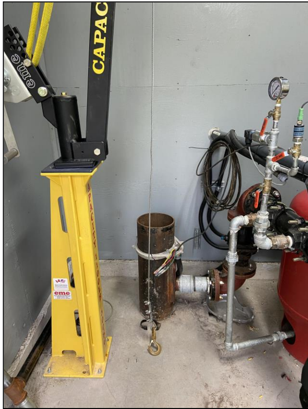
Figure 4: Well Casing in the hut
