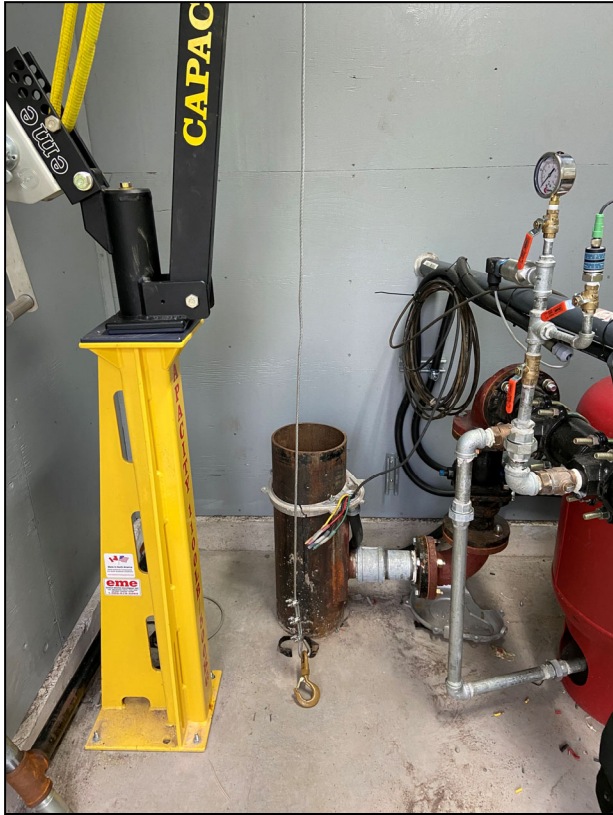
Figure 4: Well Casing in the hut
