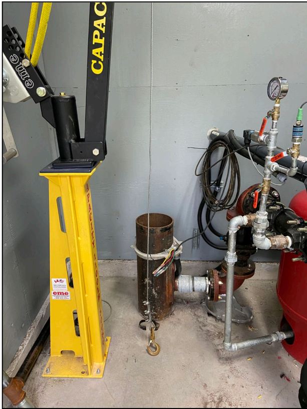
Figure 4: Well Casing in the hut
