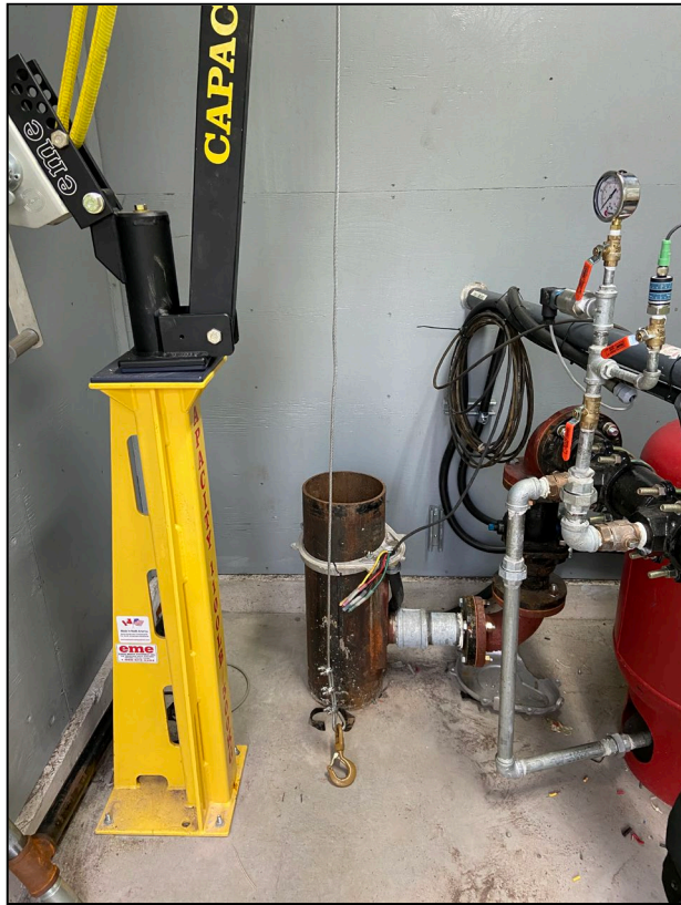
Figure 4: Well Casing in the hut
