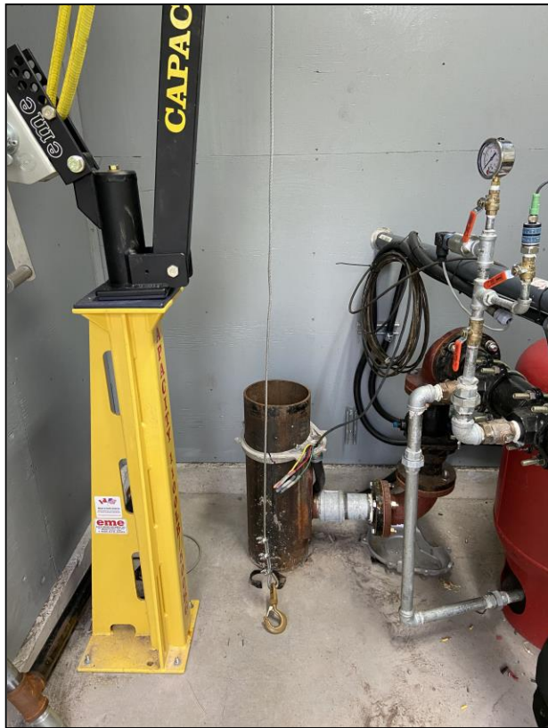
Figure 4: Well Casing in the hut
