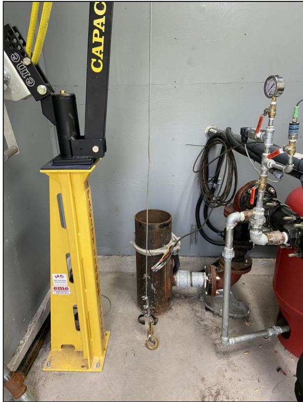
Figure 4: Well Casing in the hut
