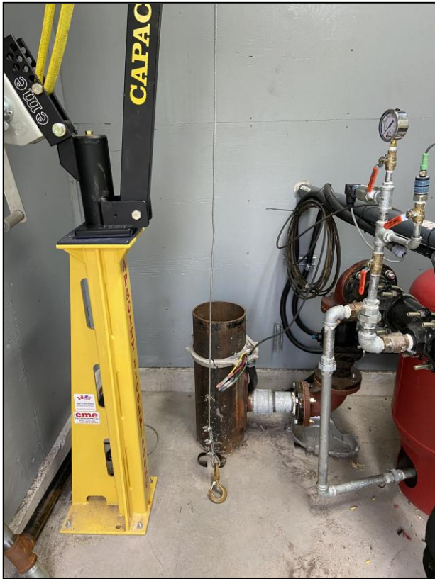
Figure 4: Well Casing in the hut
