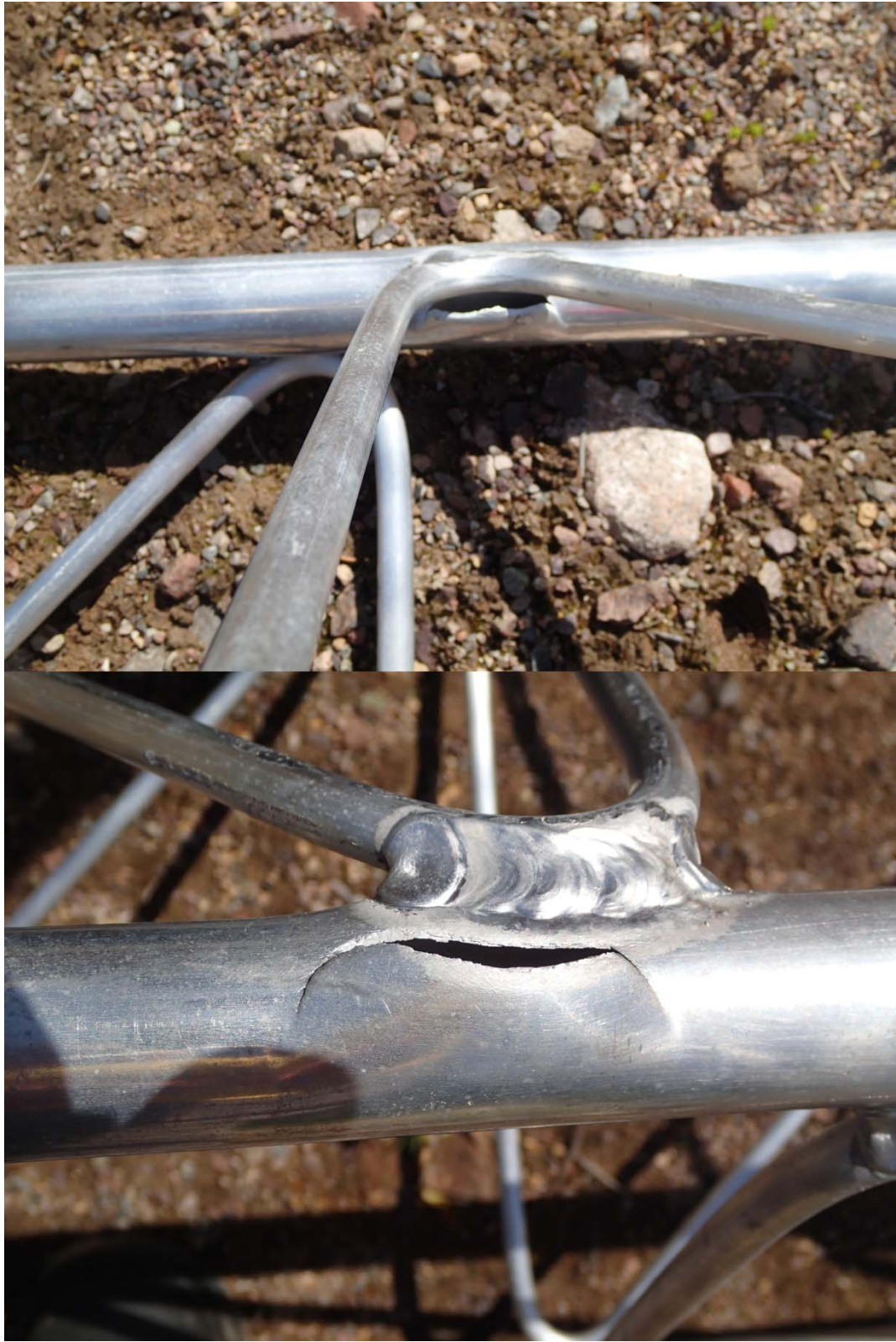
Figure 4: Compromised Tower Integrity at Sandy Lake near Birchy Narrows (Camp 55)
