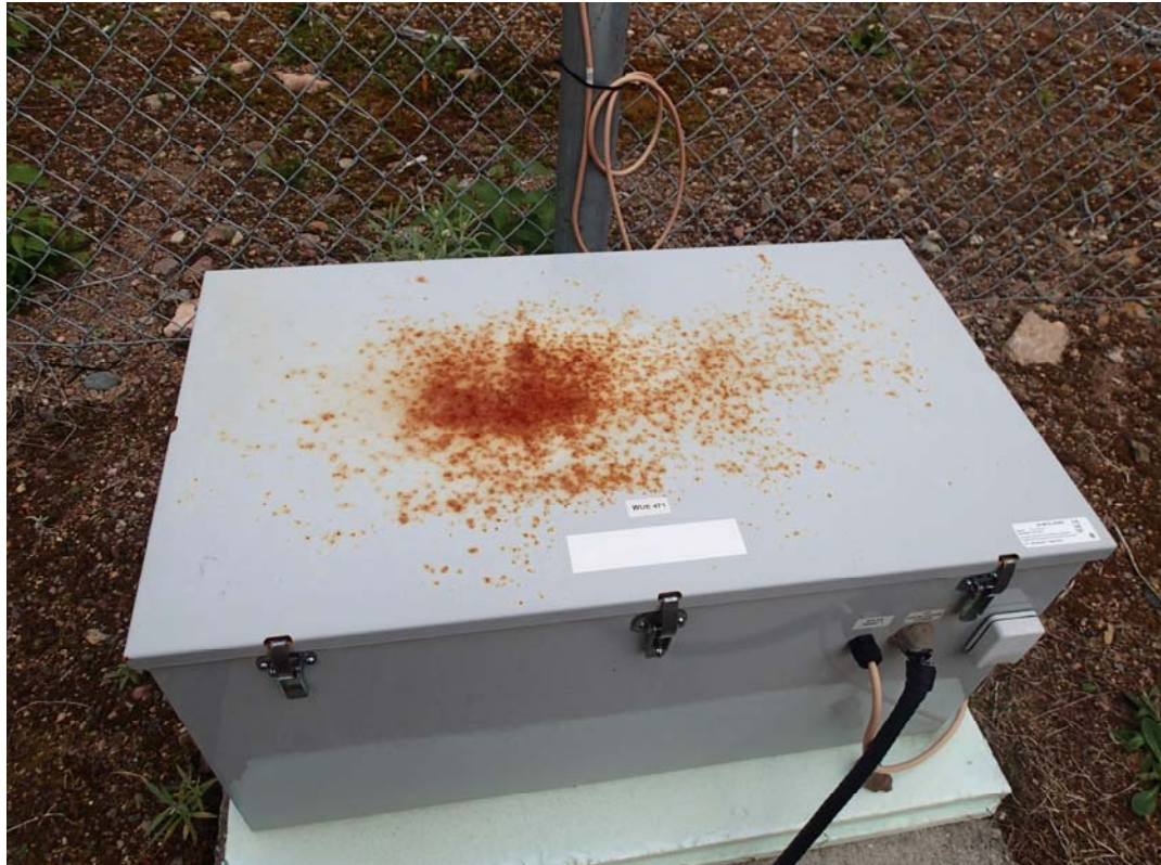
Figure 4: Battery Box Enclosure Rust conditions at Sandy Lake near Birchy Narrows (Camp 55)
