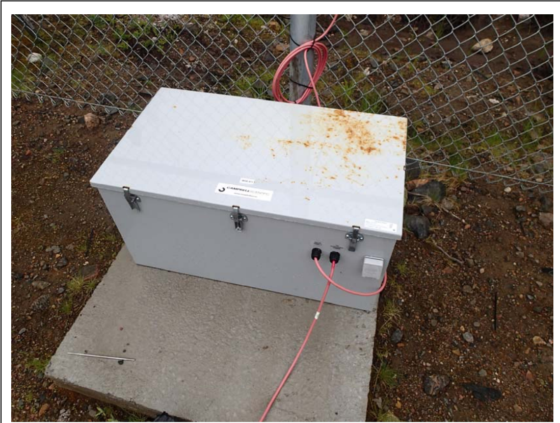
Figure 9: Battery Box Enclosure Rust conditions at Upper Humber at Black Brook
