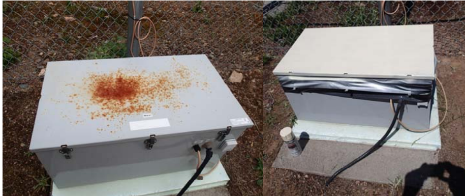
Figure 4: Battery Box Enclosure before and after maintenance at Sandy Lake near Birchy Narrows (Camp 55)
