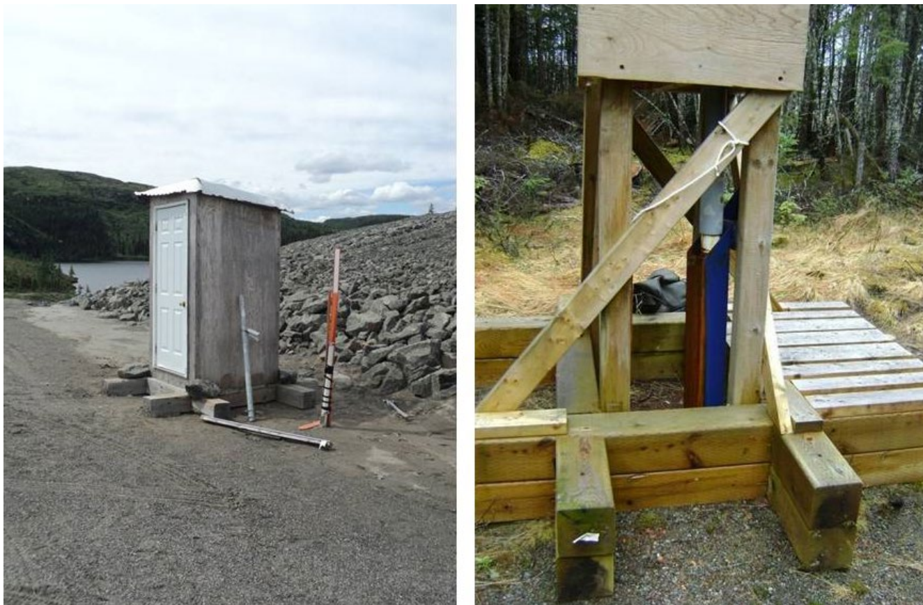
Figure 4-4: Examples of well monitoring stations
