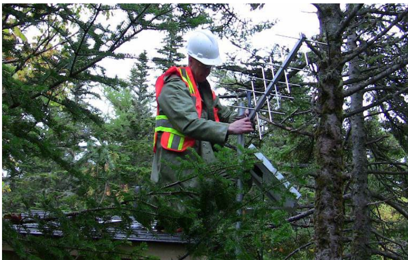
Figure 3-7: Installation of GOES antennae on a RTWQ monitoring station
