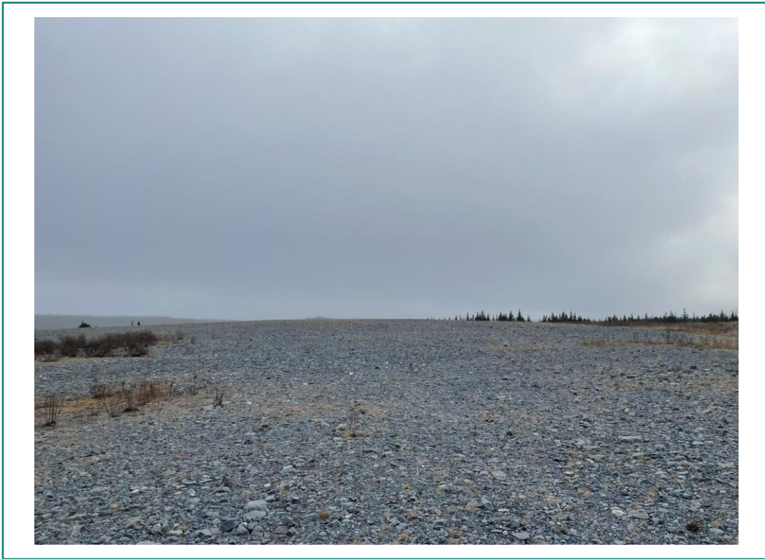
Photo 3: Overview of cap conditions at the hazardous waste landfill.
