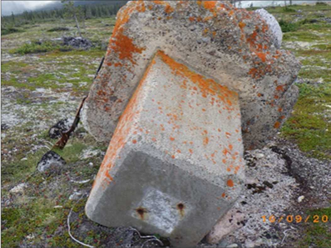
PHOTO 33 - APEC #6: Overturned concrete pillar. (September, 2017)
