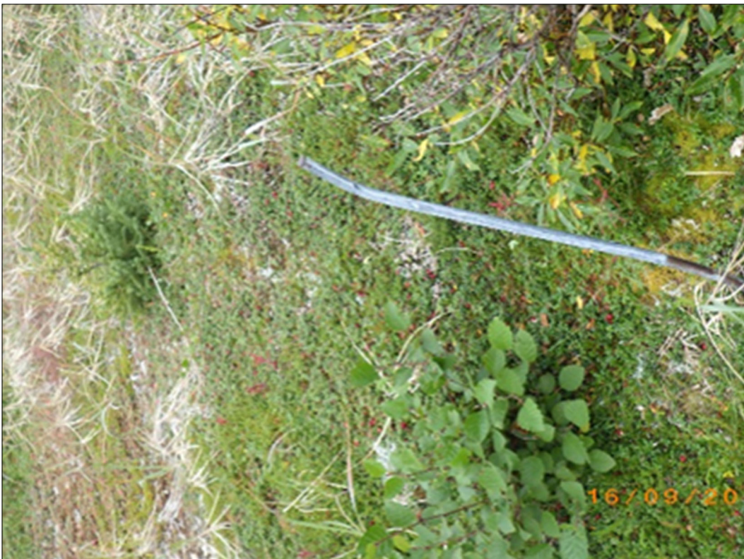
PHOTO 38 - APEC #7: Rebar coming out of the ground. (September, 2017)
