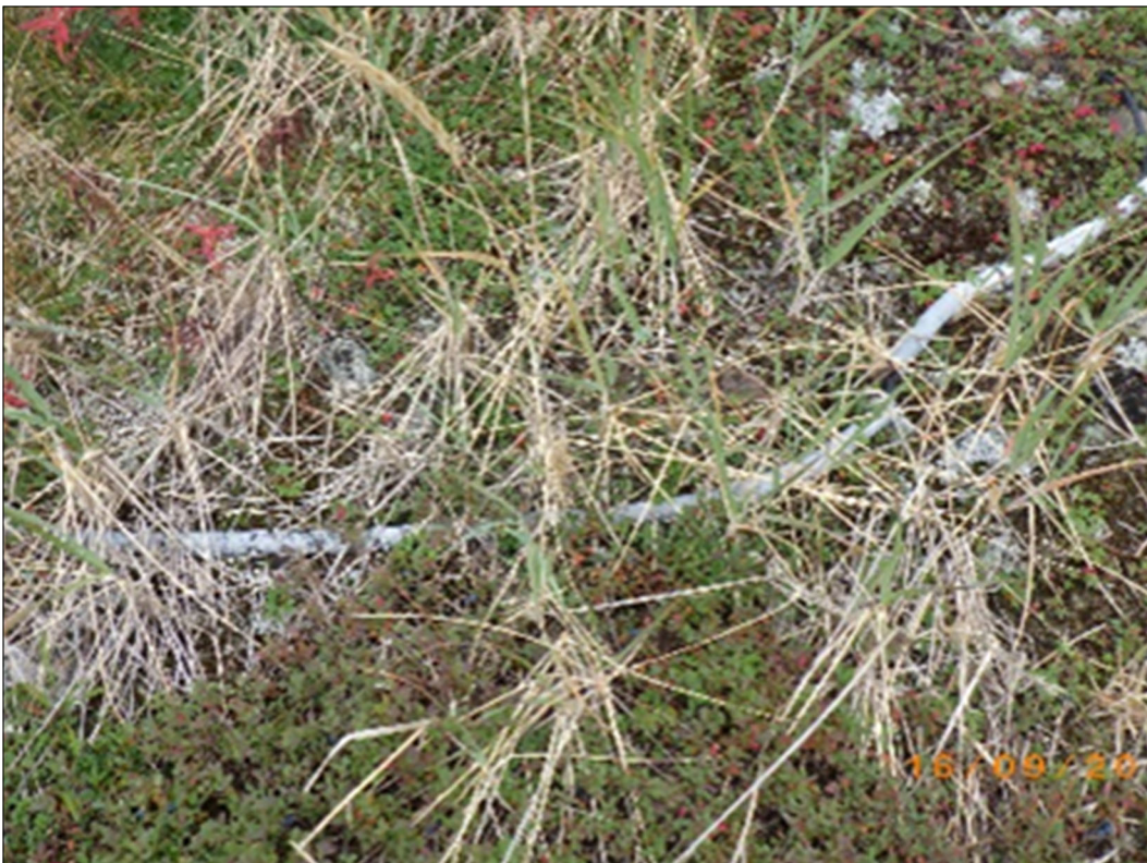
PHOTO 40 - APEC #7: Rebar coming out of the ground. (September, 2017)
