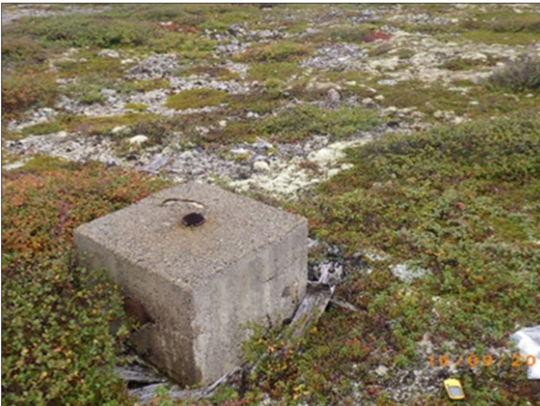
PHOTO 20 - APEC #4: Pipe going through a concrete block. (September, 2017)
