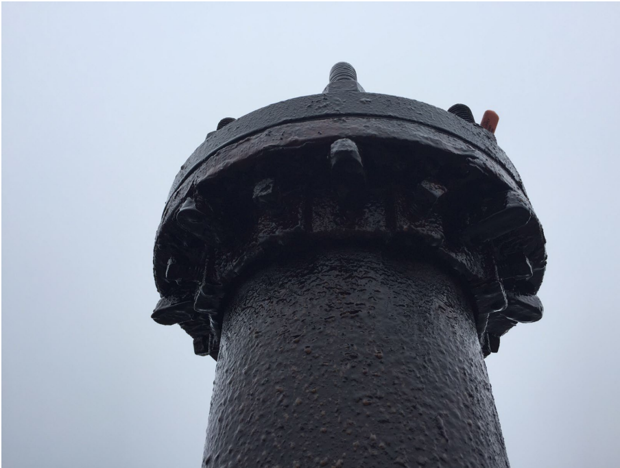
Photo 1 – Oil Coated Extension Pipe of Well Repair #1
