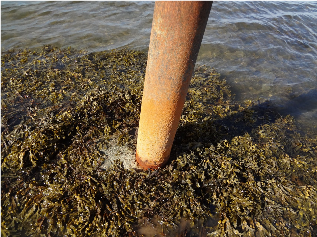
Photo 2 – Seaweed on Concrete Base of Well Repair #1
