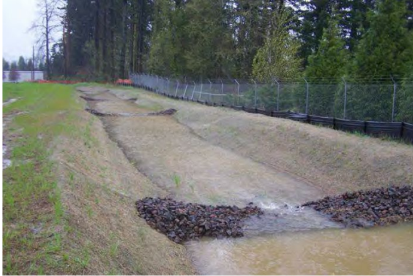
Figure 8: Grass-lined swale with check dams (Erosion Prevention and Sediment Control Planning and Design Manual, 2020)
