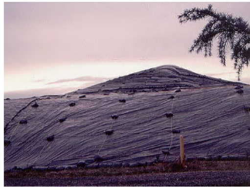
Figure 13: Plastic sheeting over a slope (Erosion Prevention and Sediment Control Planning and Design Manual, 2020)
