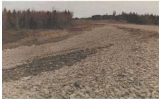
Figure 14: Riprap lining for an embankment (Erosion and Sedimentation Control - Handbook for construction site)
