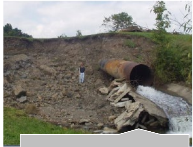
Another dam failure due to internal erosion
