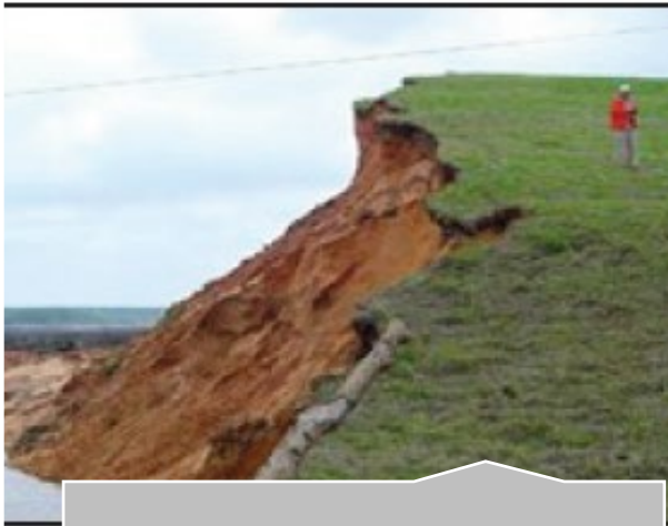
Failure of dam due to internal erosion
