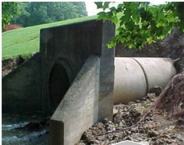
Internal Erosion along concrete pipe
