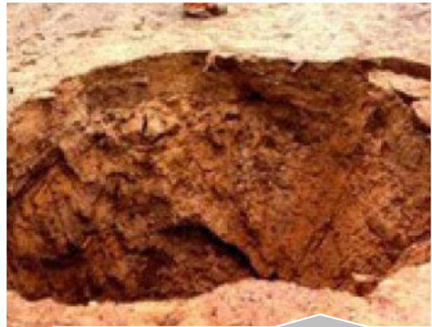
Sinkhole as a result of internal erosion
