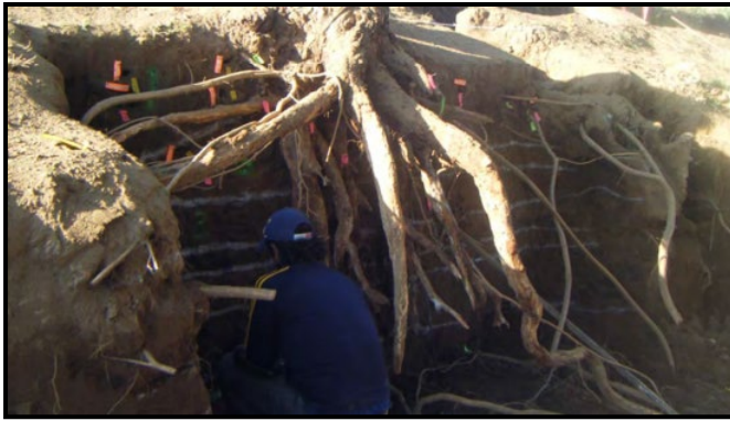
Figure 6 – Eucalyptus tree root system within embankment slope exposed Image retrieved from (Shriro, et al., 2013, Pg. 97)
