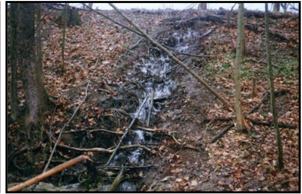
Figure 7 - Seepage caused by piping through a dam's embankment. (United States Department of Agriculture, Pg. 13).
