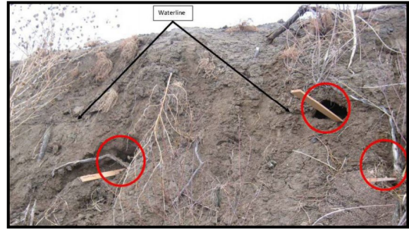
Figure 5 – Muskrat burrows accompanied by tree roots on an earthen slope. Three burrows, initially marked by pieces of wood, are indicated with red circles. A waterline appears to intersect the upmost burrow entrance, and fall above the other two burrows. Retrieved from Hahn et al (n.d.), slide 85.
