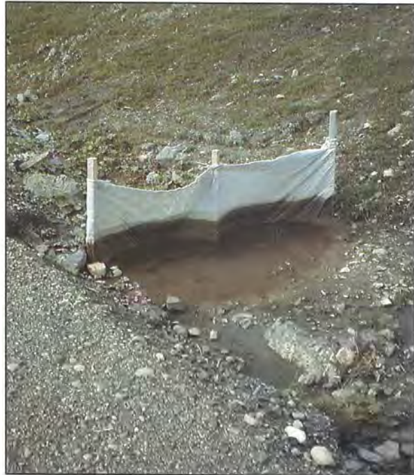
Failure to key the dam into the ditch sides allowed water to wash around the dam.
