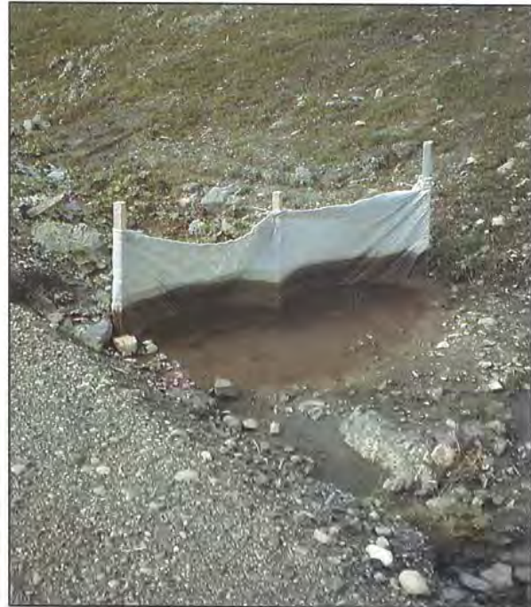
Failure to key the dam into the ditch sides allowed water to wash around the dam.
