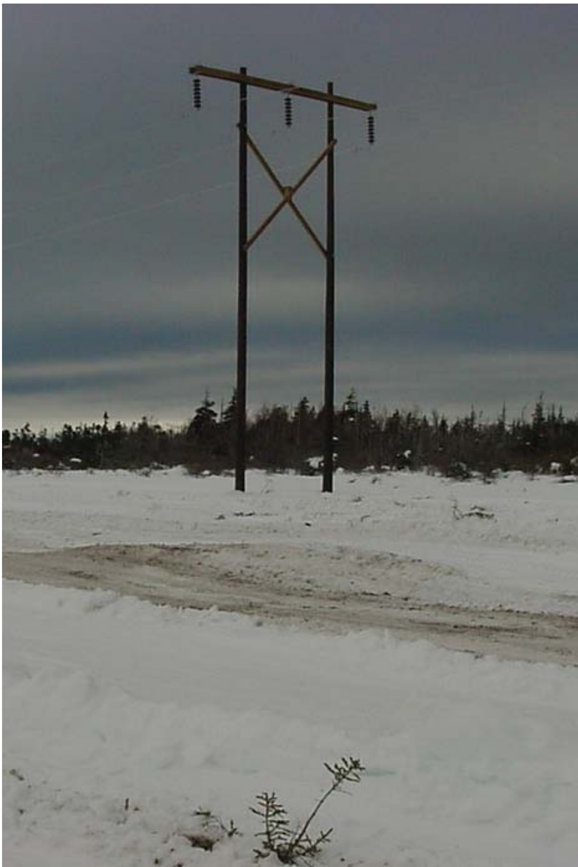
Figure 8: Example of a 66 kV standard “H Frame Structure”.
