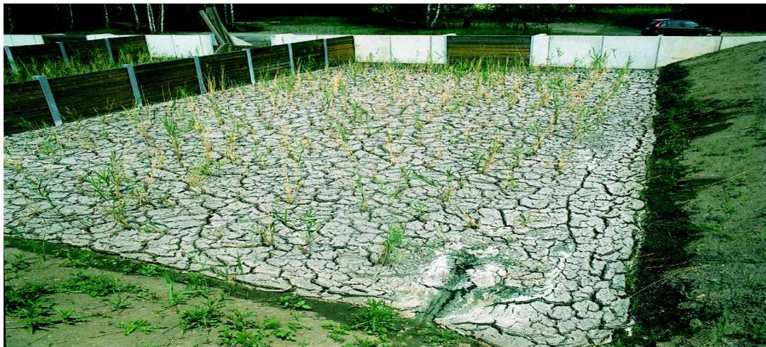
Figure 10 Completed solids treatment facility
