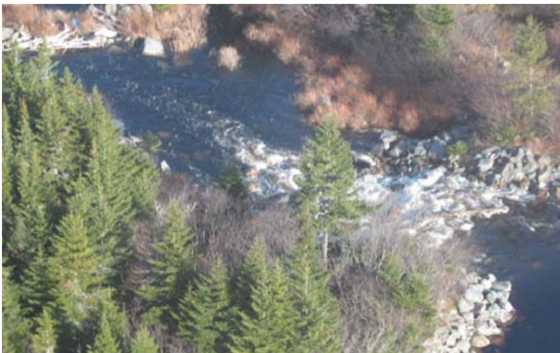
Figure 9.4 Rock-fill dyke at the outflow of Sam Howe's Pond (P14) during high flow, January 8, 2007.
