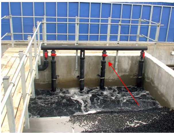
Picture 17 Example of a moving bed filter. Red arrow indication the valves for regulation of air flow
