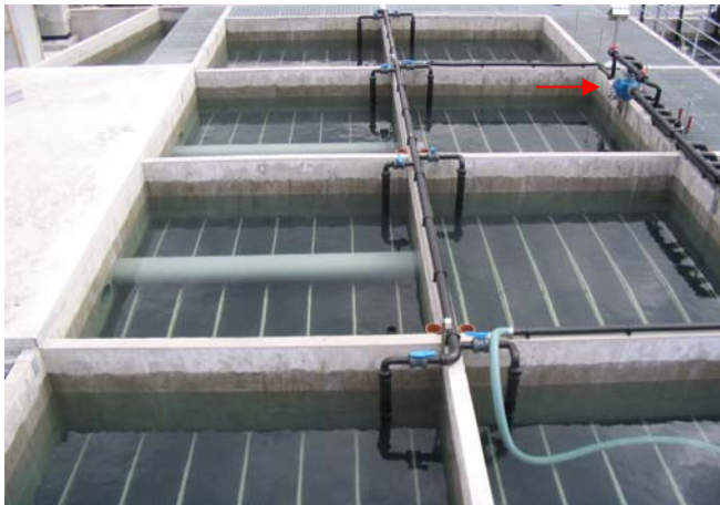
Picture 14 Example of “fixed bed” biofilter.
