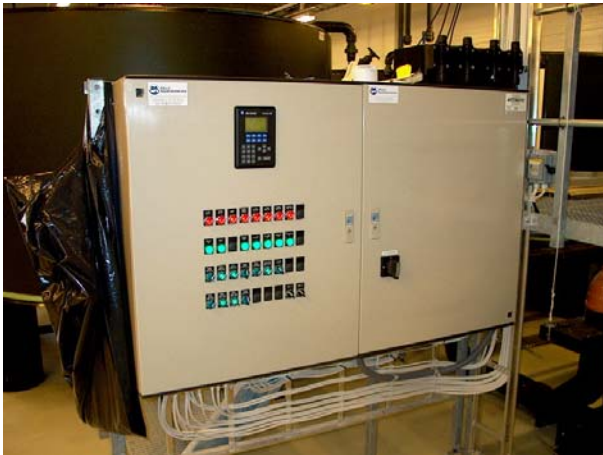
Picture 29 Power cabinet with PLC
