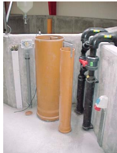
Picture 2 Example of a stand pipe
