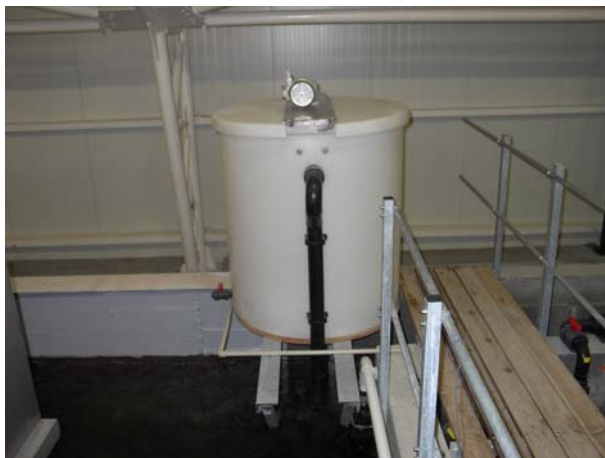
Picture 26 Lime dosing
