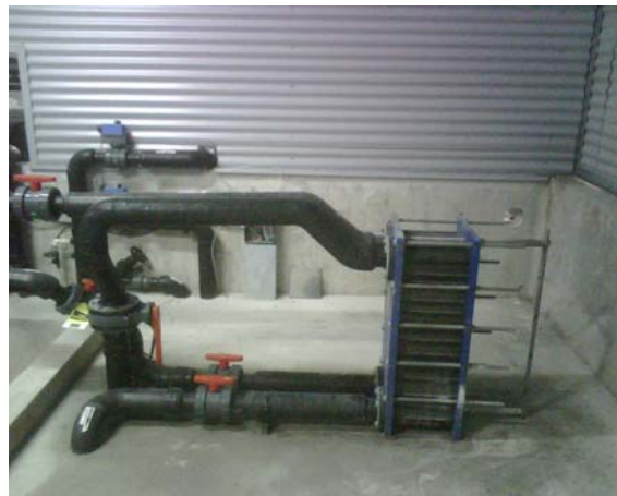
Picture 28 Heat exchanger
