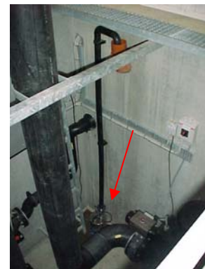
Picture 13 Pump for empty the pump sump
