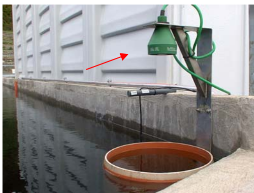
Picture 8 Ultra sensor by the drum filter
