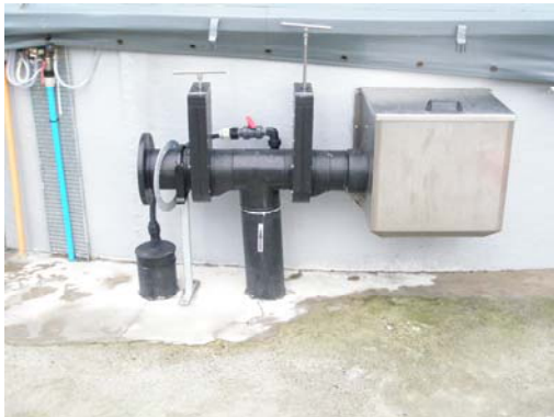
Picture 5 Connection for fish pump
