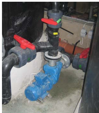
Picture 25 Example of discharge water pump
