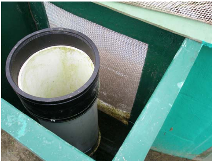
Picture 1 Example of a side drain
