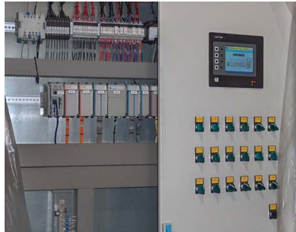
Picture 30 Power cabinet with PLC and touch screen
