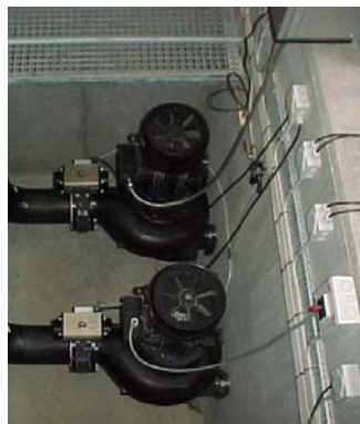
Picture 12 Centrifugal pumps in pump sump
