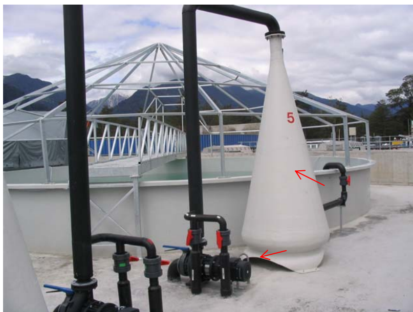
Picture 21 Example of pump and cone connected to each tank
