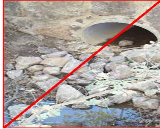
Figure 5-32: Incorrect Construction of Rock Energy Dissipaters
