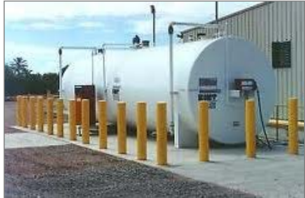
Figure 5-6: Fuel storage on concrete pad
