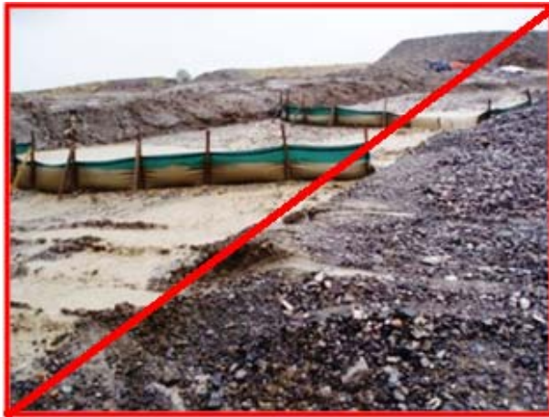
Figure 5-36: Examples of poorly installed silt fences
