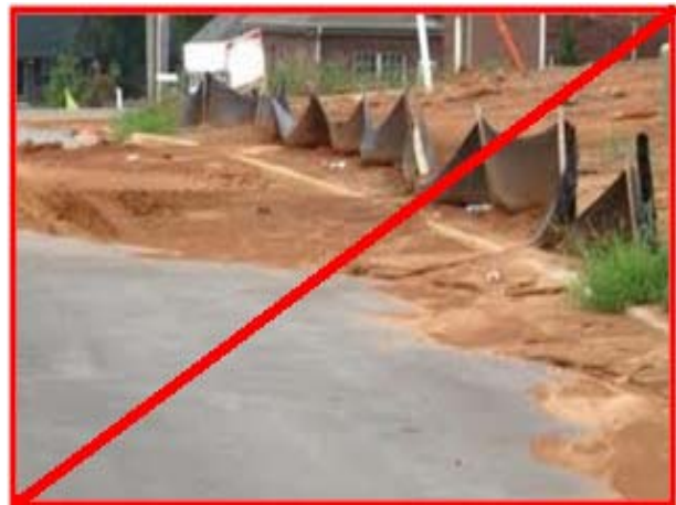
Figure 5-37: Examples of poorly installed silt fences
