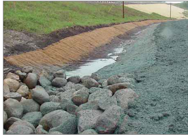
Figure 5-26: Photograph shows erosion control blanket on slope and erosion control mat in channel
