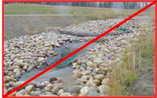
Figure 5-28: Photograph of failed Rip Rap Protection
