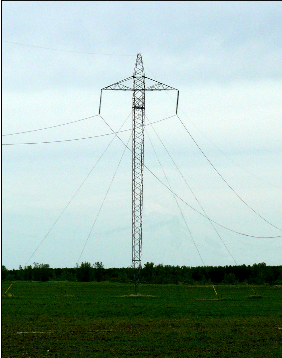
Figure 2.5 Typical HVdc Transmission Tower
