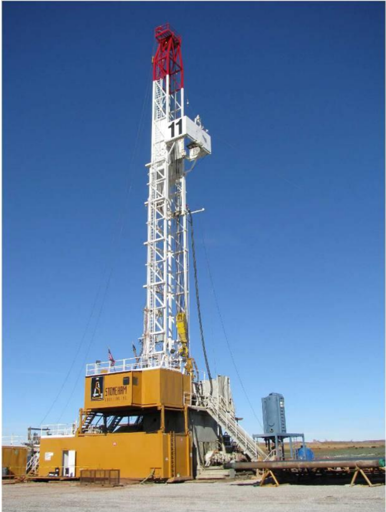
Figure 3-4 Photograph of a Typical Drilling Rig (Example of an Operating Rig and Well)
