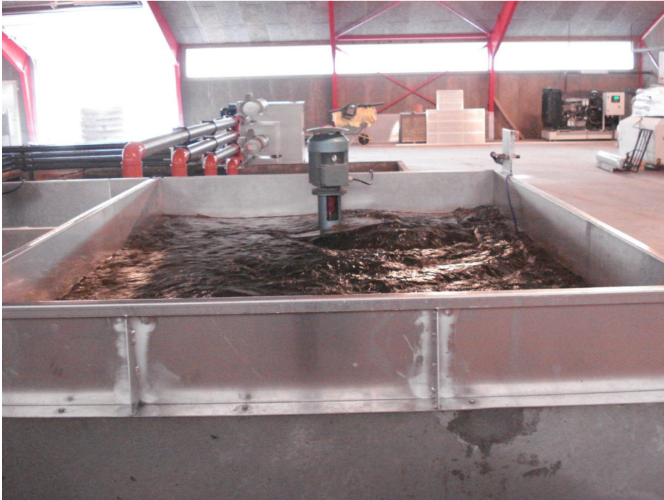
One of the two injector platforms for adding liquid oxygen to the water
