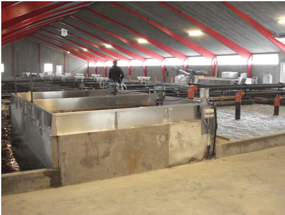
The rearing unit with the aeration area and injector platforms in the foreground
