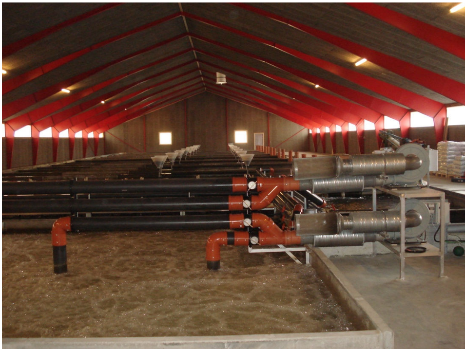
Degassing with Ventur blowers and pipe system
