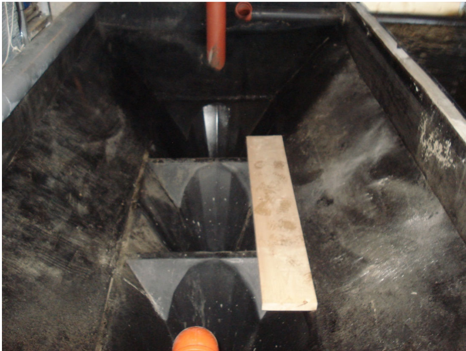
Sludge treatment for sludge water from microsiew
