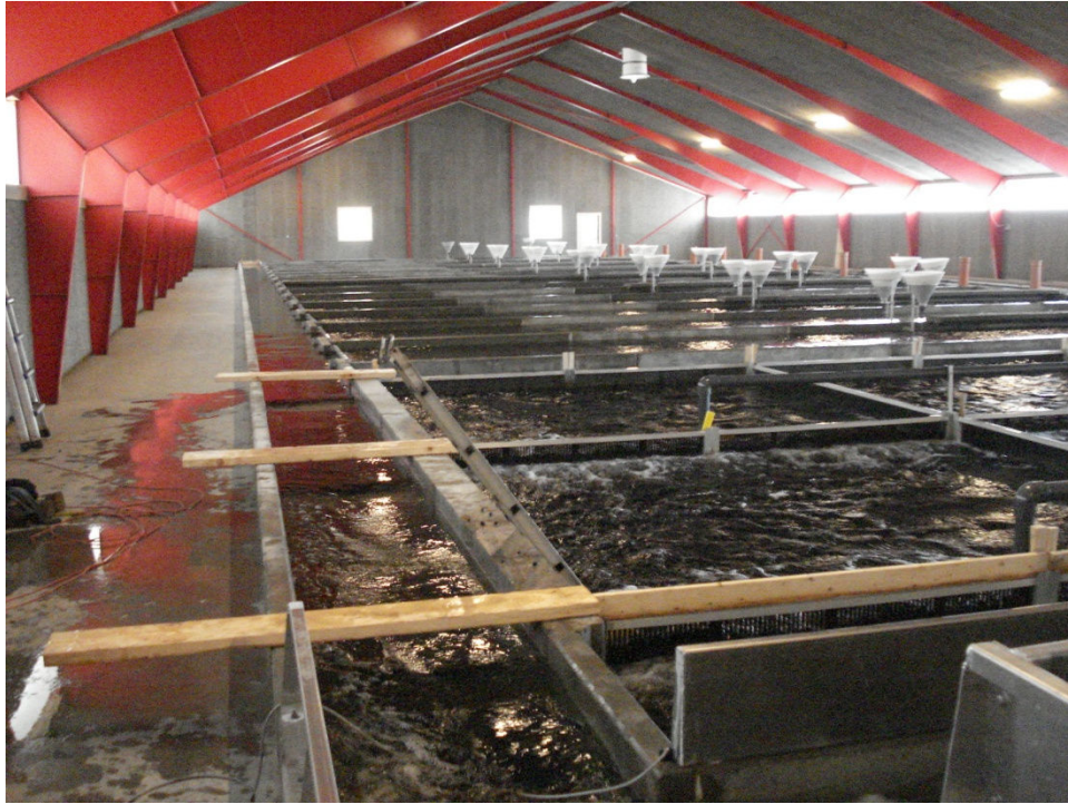
The system seen from the south end of the building, with the biological filter in the foreground
