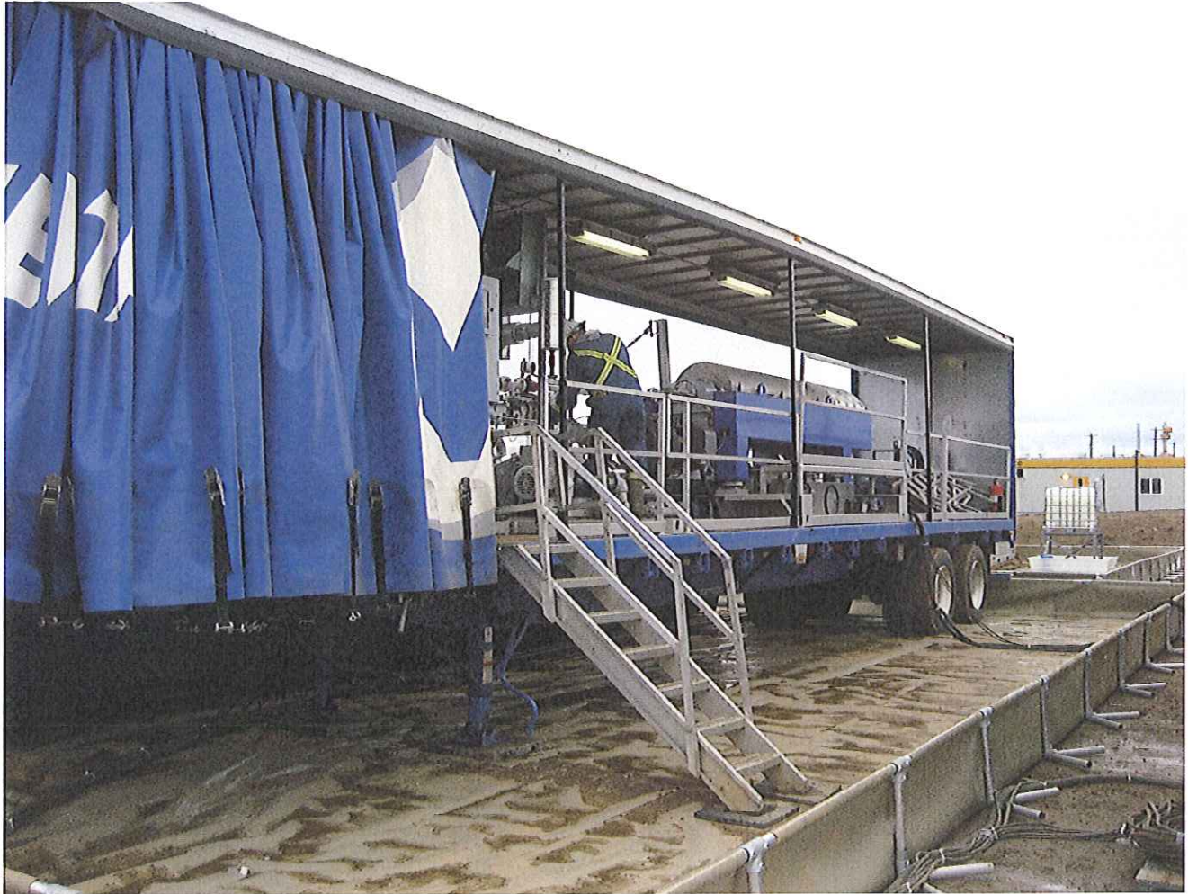
Figure 5 centrifuge trailer set-up inside secondary containment.
