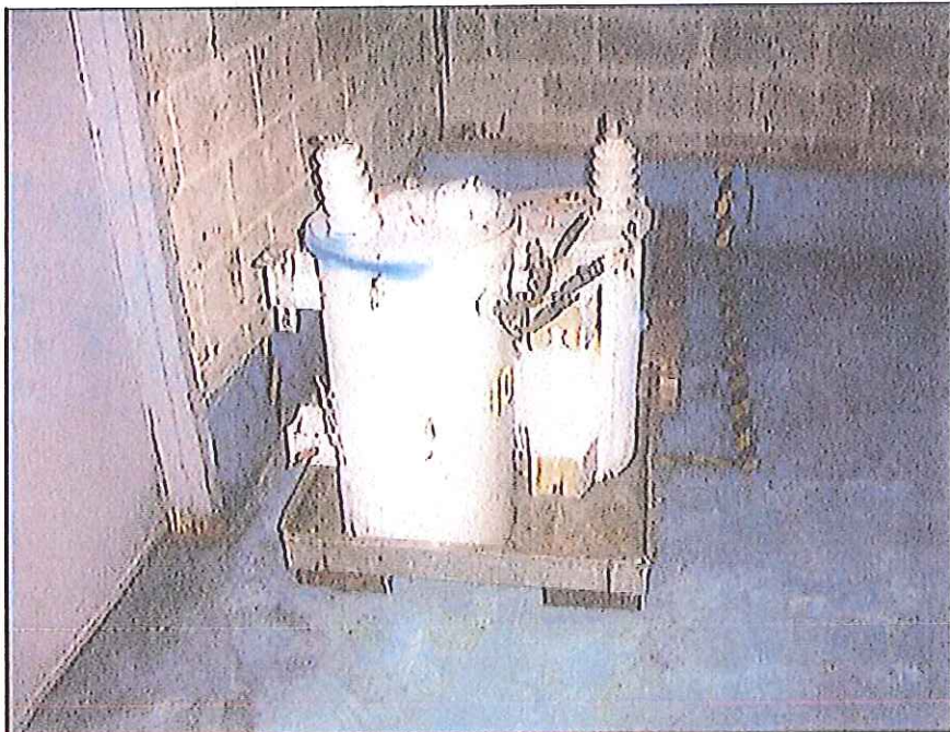
PCB-containing transformers in warehouse.
