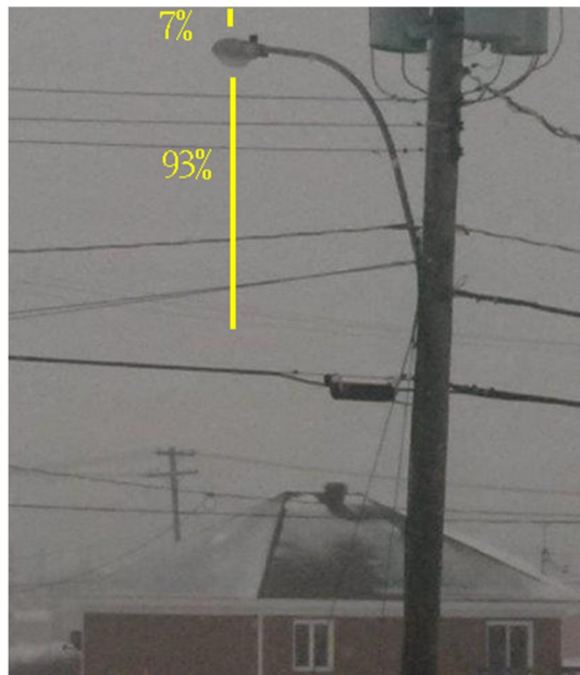
Figure 3 Cobrahead fixture typically used in the Schefferville area
