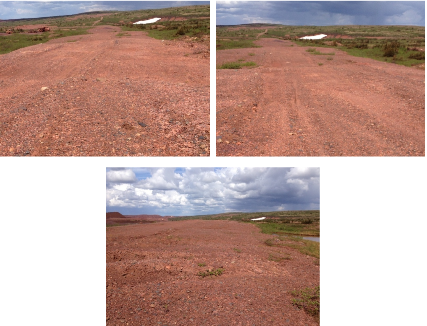
Figure 4-3: Photos of Degradation of Permafrost over 50 Years on old Fleming Haul Roads
