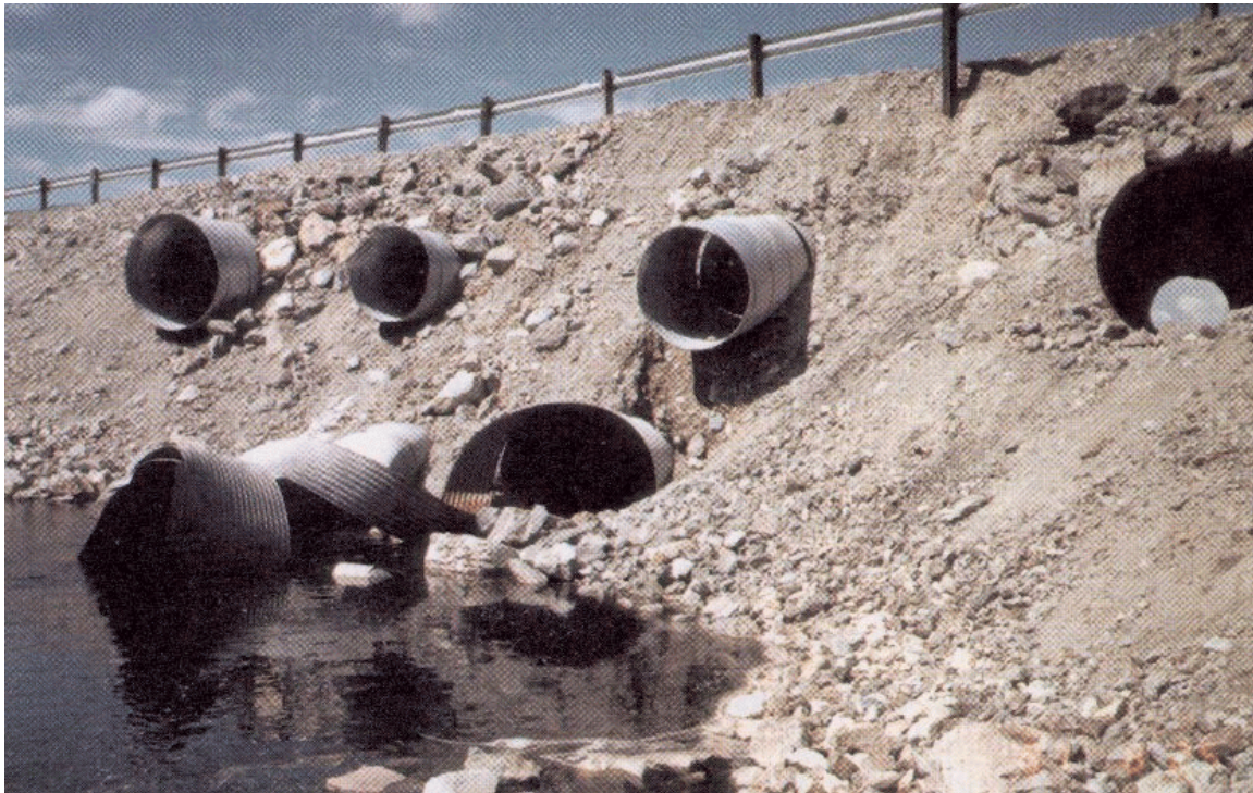
Figure 5.5 Poorly Installed Culverts
