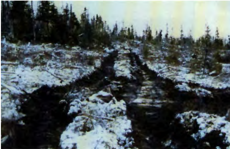
Figure 4.42 Mudlogs divert water off of the trail and onto the forest floor.
