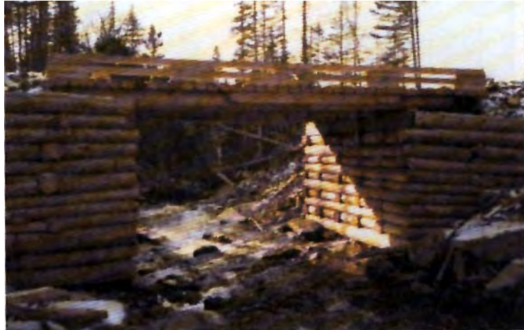
Figure 4.16 Untreated or pressure treated wood should be used for timber crib construction.
