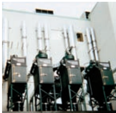
Gold Series® installation on weld smoke
