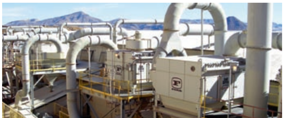
GS units on crushing copper ore
