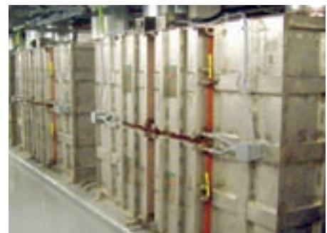
HEPA's after dust collectors
