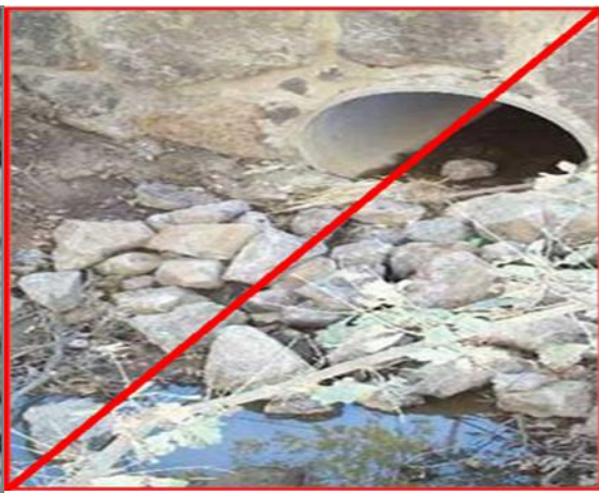
Figure A-12 - Incorrect Construction of Rock Energy Dissipaters
