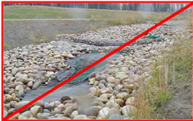
Figure A-8 - Photograph of failed Rip Rap Protection a Slope
