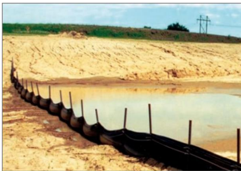
Figure A-13 - A Well Constructed Silt Fence
