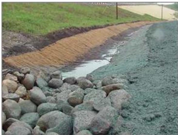
Figure A-6 - Photograph Shows Erosion Control Blanket on Slope And Erosion Control Mat in Channel
