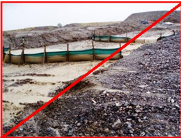
Figure A-16 - Examples of Poorly Installed Silt Fences
