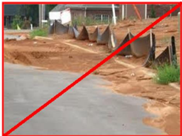
Figure A-17 - Examples of Poorly Installed Silt Fences
