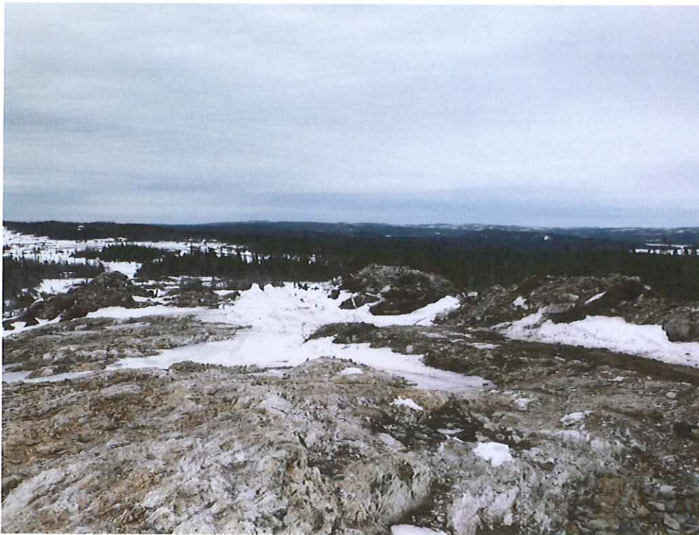
Figure 7. Same trench as in Figure 6. Note that the excavated piles contain organic cover (dark) which should have been separately stockpiled.
